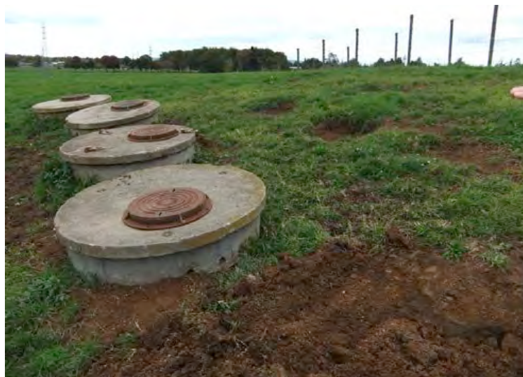
Figure 8: Carcass pit covers and subsidence holes
