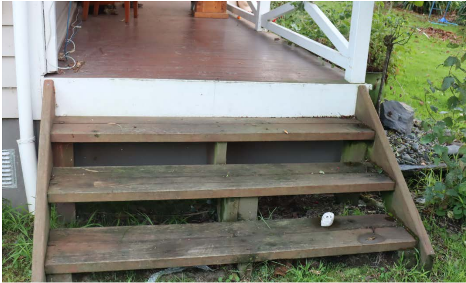
Stairs Not original
