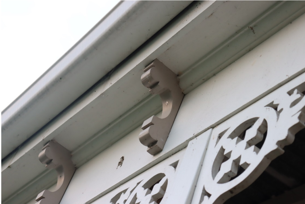
Not original – had made and fitted with stainless steel screws
