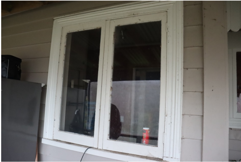
Wash house and kitchen windows both not original
