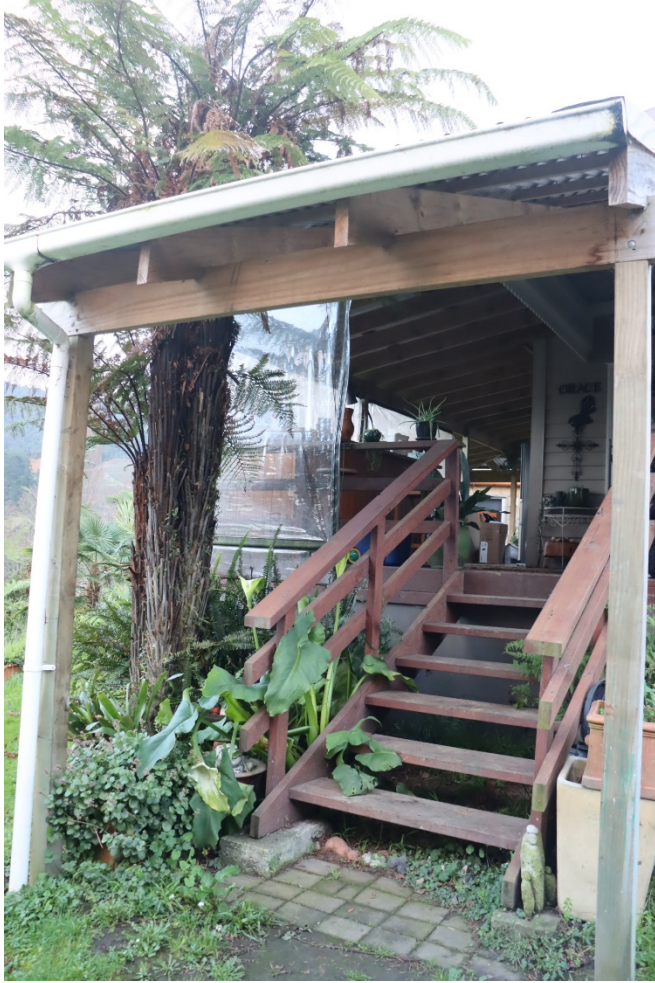
Stairs, deck and awning not original
