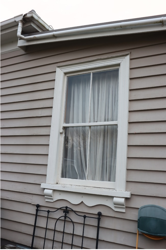
Decorative work below window not original
