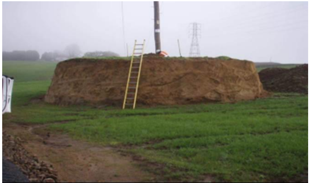
Figure 4: NZECP34 compliant earthworks around a pole on ARI-HAM-A 110kV pole line off Orepunga Road (Karāpiro)
