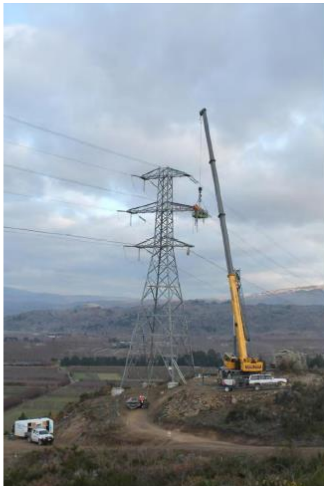
Figure 16: Example crane access required for cross arm and insulator works as part of re-conductoring
