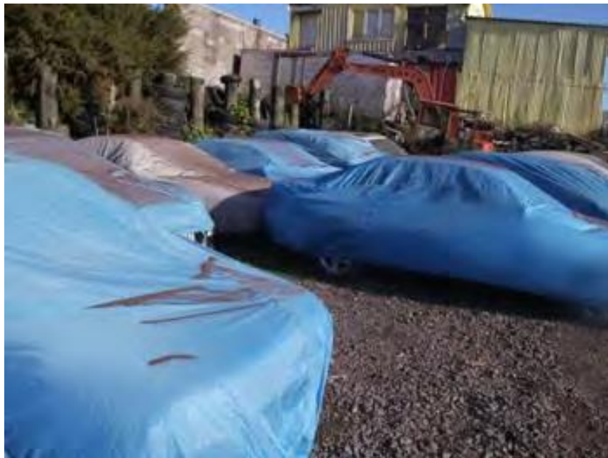
Figure 6: Tower painting in an industrial setting showing garnet debris falling onto cars
