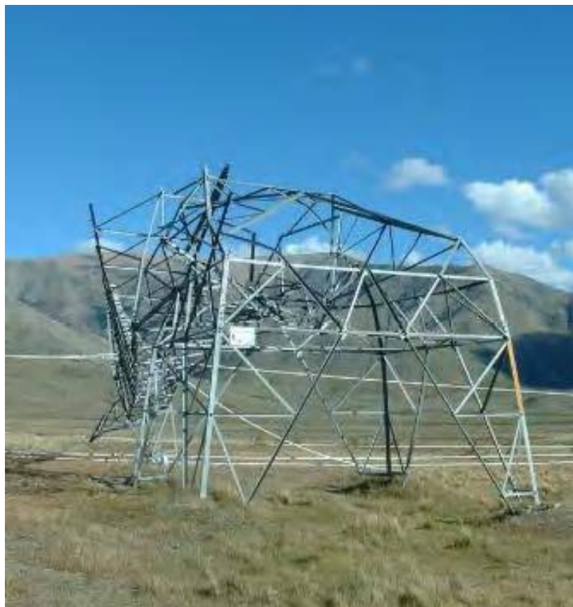
Figure 19: Failed tower on the Benmore-Haywards A line
