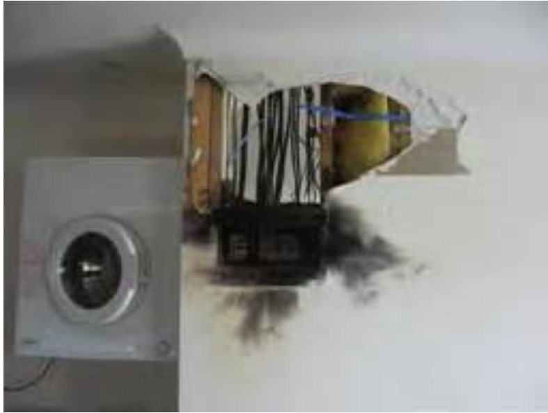
Figure 17: Electrical damage following a conductor drop
