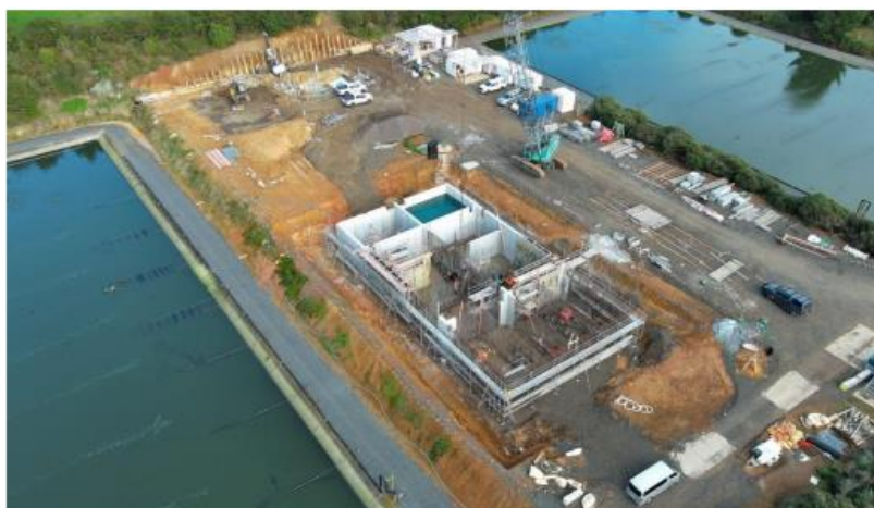
Raglan WWTP MBR Upgrade– The reactor tank foundation is complete and the wall installation is underway.
