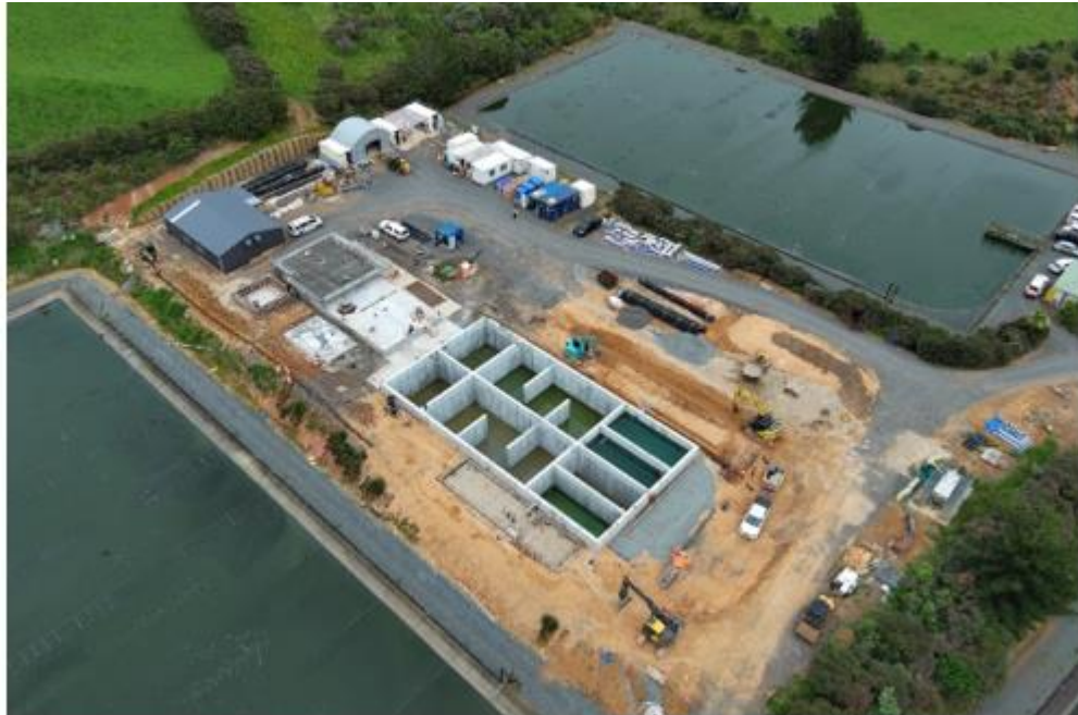
Raglan WWTP MBR Upgrade - The reactor tank, inlet works platform, and new plant building.
