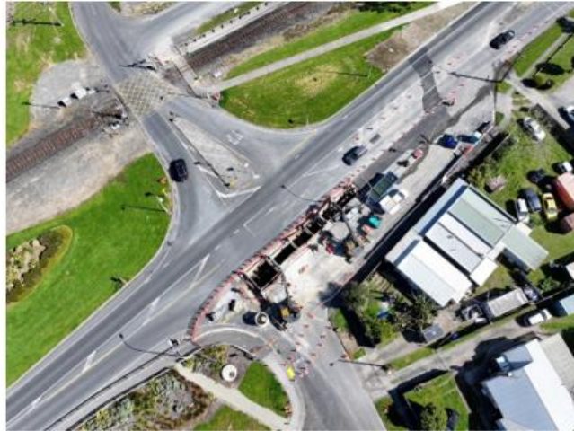
Ngaaruawaahia Pipeline – Regent St, installation of the last section of the gravity sewer.
