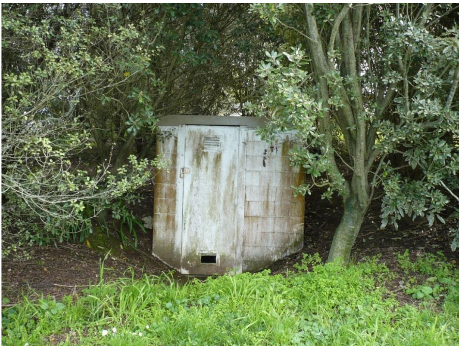
Figure 5 Western District Zone Booster Pump Station
