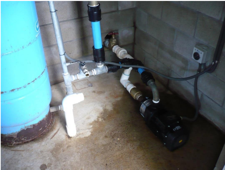
Figure 8 Western District Zone Booster Pump
