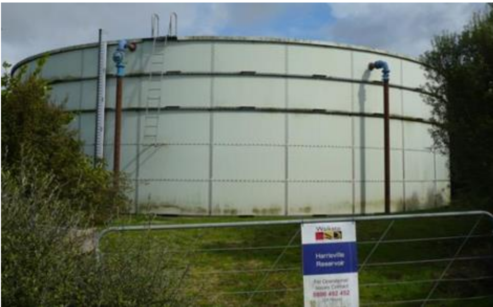
Figure 6 Harrisville Road Steel Reservoir
