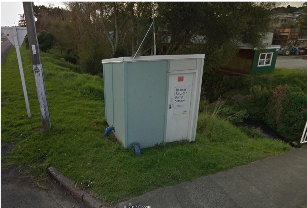
Figure 10 Railway Booster Pump Station
