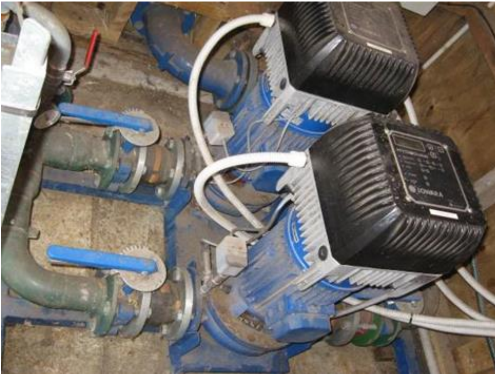
Figure 11 Railway Booster Pumps
