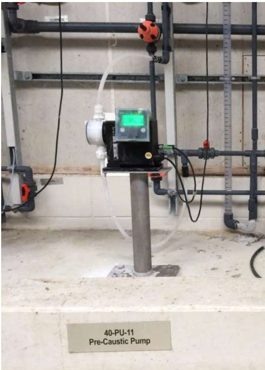
Figure 10. Pre-Caustic Dosing Equipment
