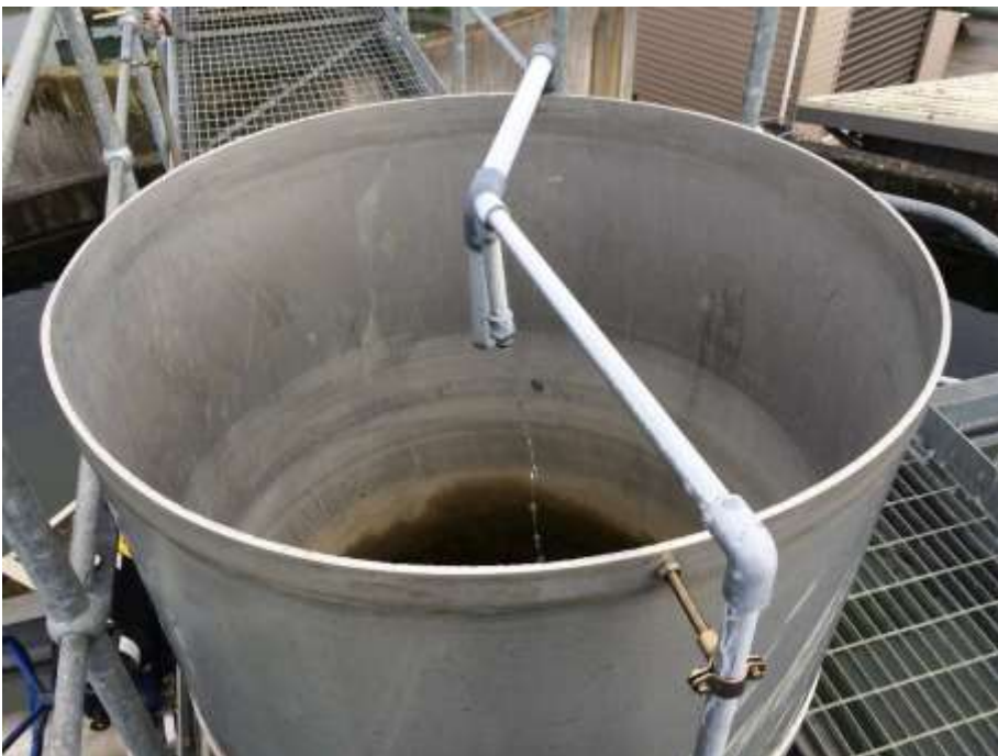
Figure 15. Clarifier Flocculation Tank, and Poly Dose Point
