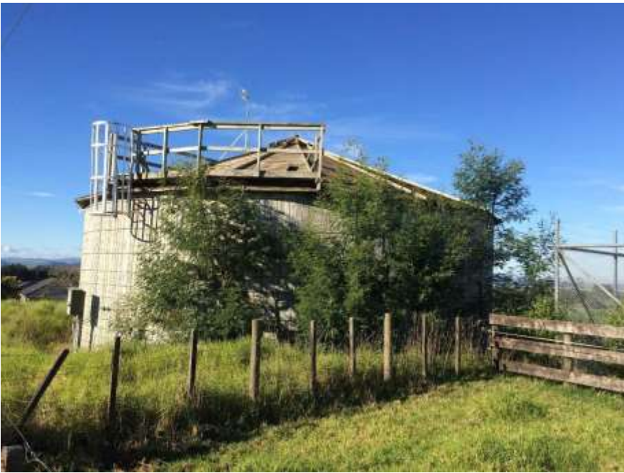
Figure 34. Network Reservoir, Te Kauwhata Road, Te Kauwhata
