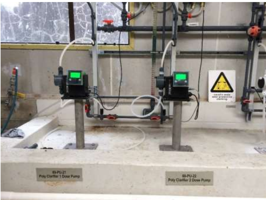
Figure 14. Poly Dosing Equipment
