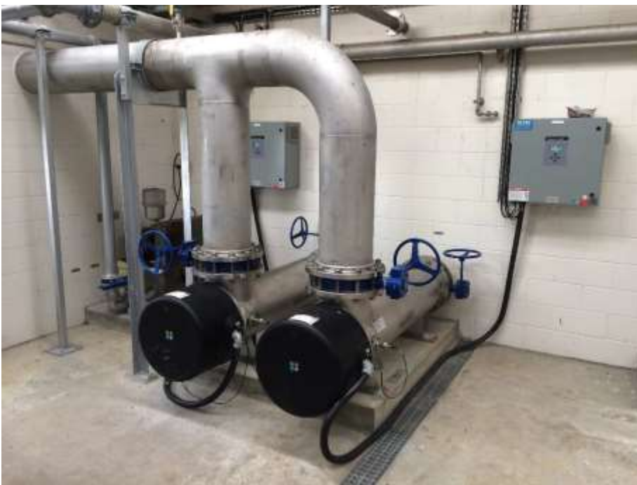
Figure 24. UV Dosing Equipment
