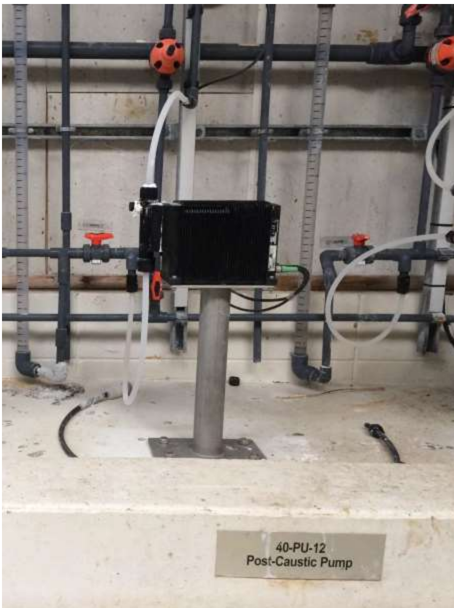
Figure 22. Post-Caustic Dosing Equipment
