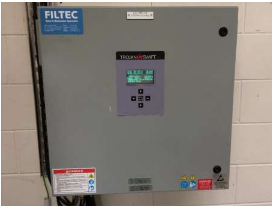
Figure 25. UV Dosing Control and Monitoring Equipment
