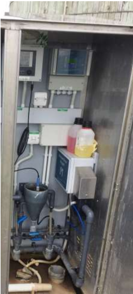
Figure 13. Coagulant and pH Dosing Monitoring Equipment
