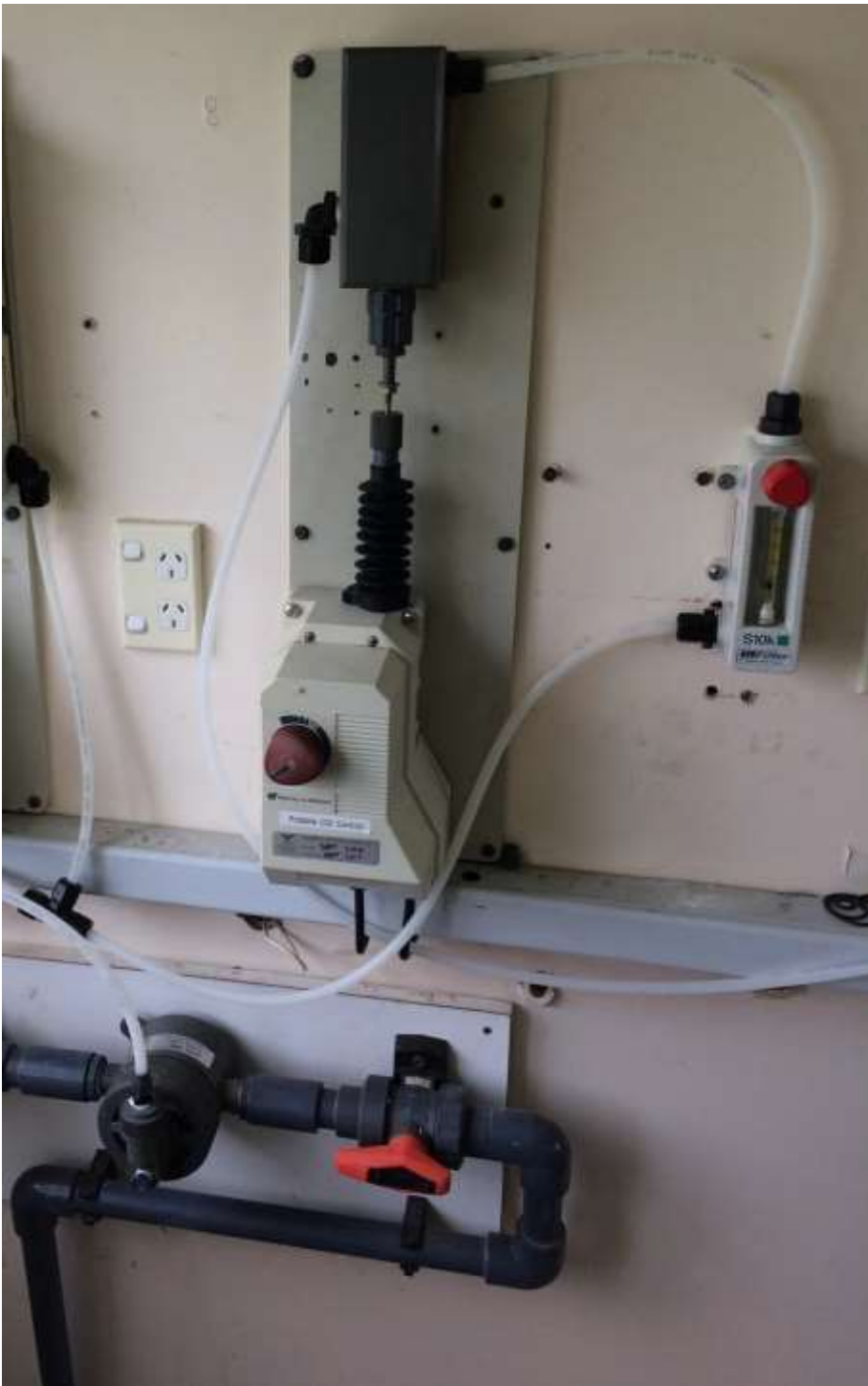
Figure 26. Chlorine Dosing Equipment
