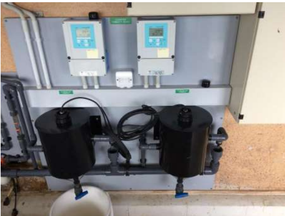
Figure 17. Clarified Water Turbidity Meters
