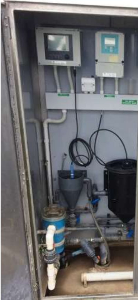
Figure 9. Raw Water pH and Turbidity Monitoring
