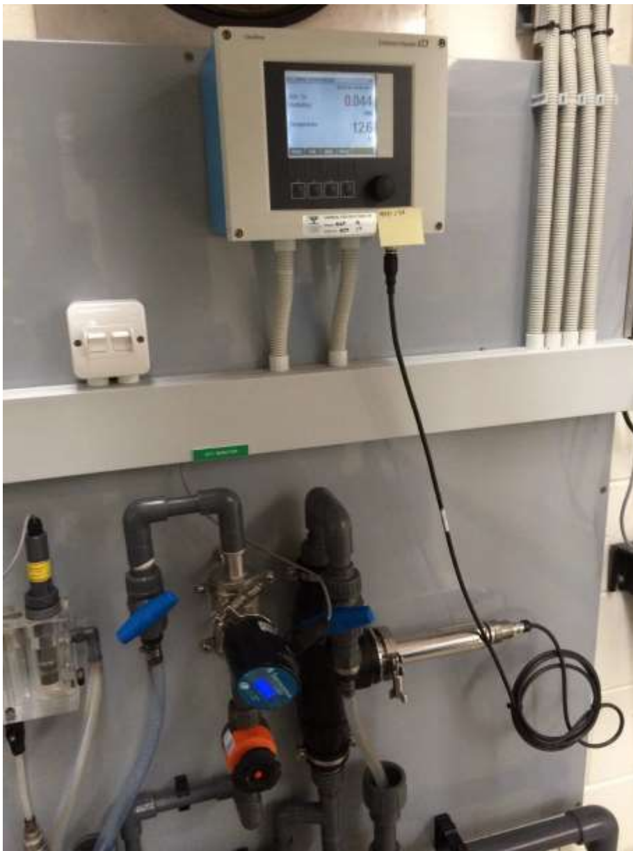
Figure 23. UVT Monitoring Equipment
