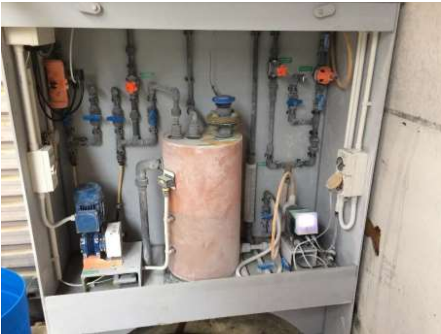
Figure 18. Fluoride Dosing Equipment
