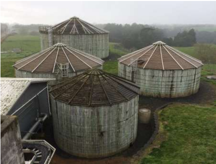
Figure 28. Backwash, and Treated Water Reservoirs
