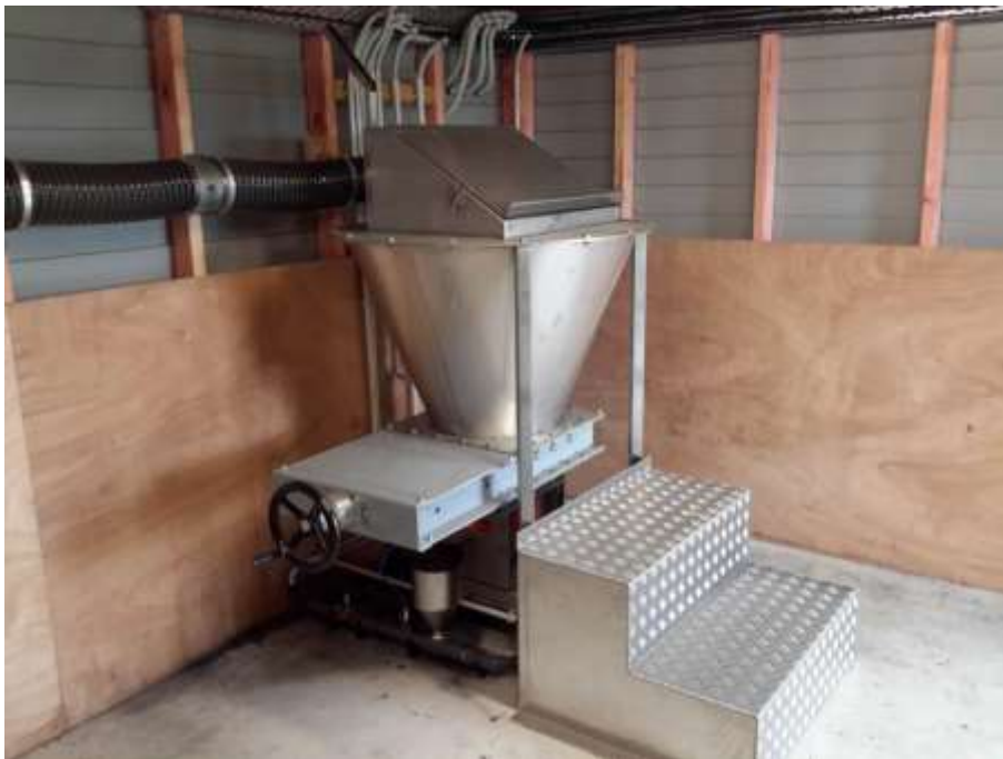
Figure 12. PAC Dosing Equipment
