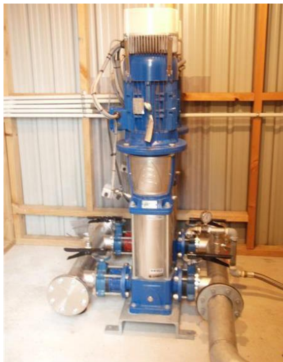
Figure 3. Newstead Reservoir Pumps
