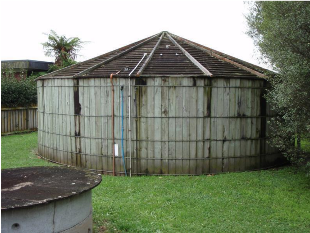
Figure 4. Matangi Road Reservoir
