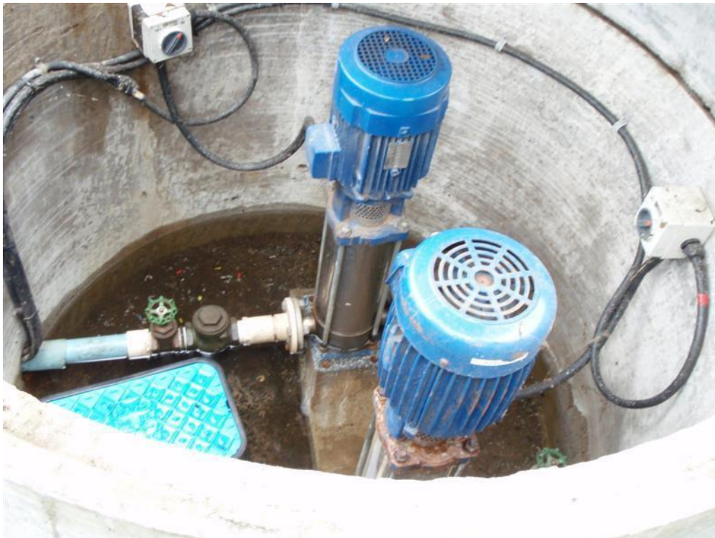
Figure 5. Matangi Road Pumps
