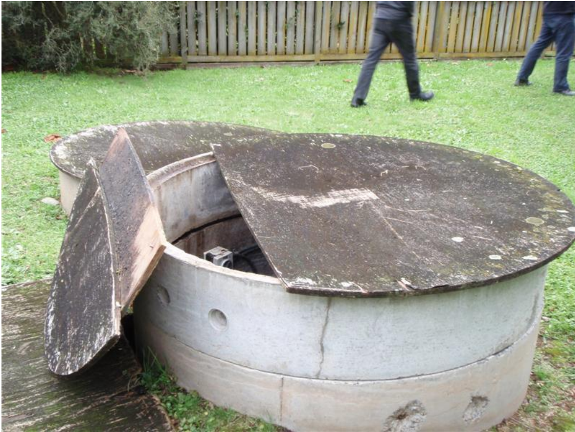
Figure 6. Matangi Road Reservoir Pump Chamber
