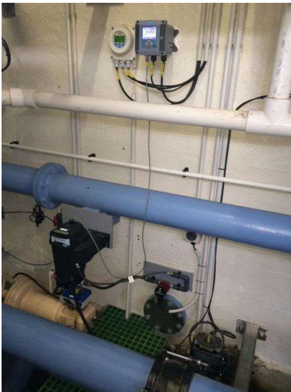
Figure 10. Individual Filter Turbidity and Flow Monitoring Equipment
