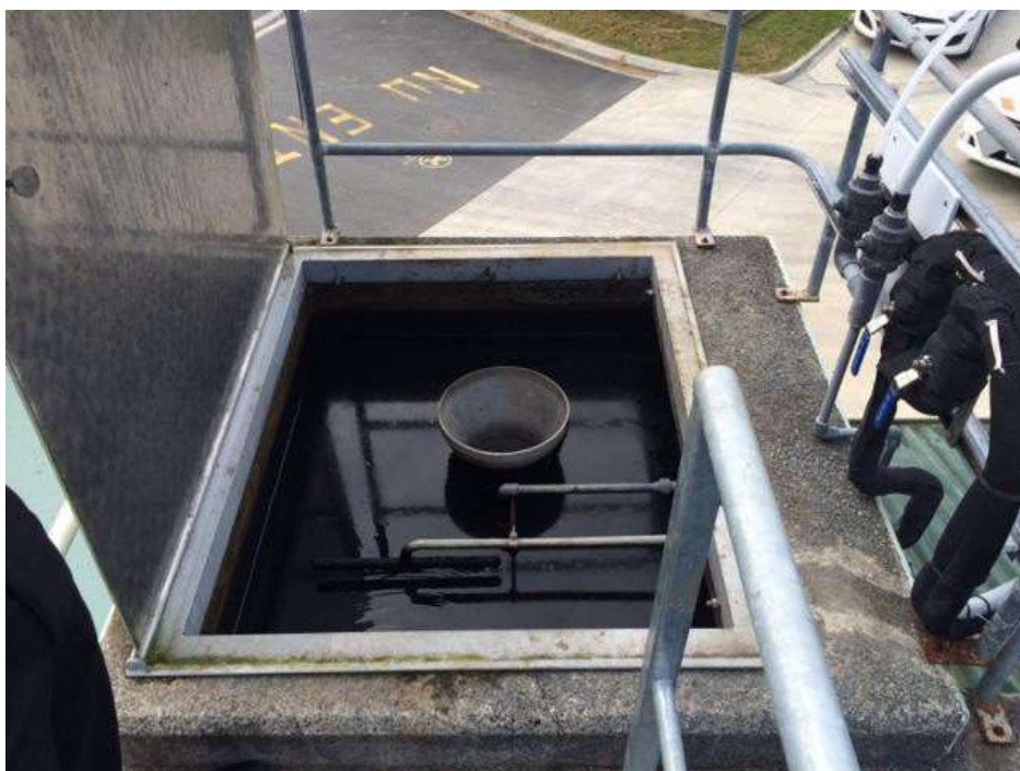
Figure 4. Flash Mixer Tank
