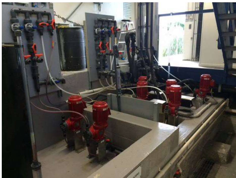
Figure 6. Coagulation Dose Pumps
