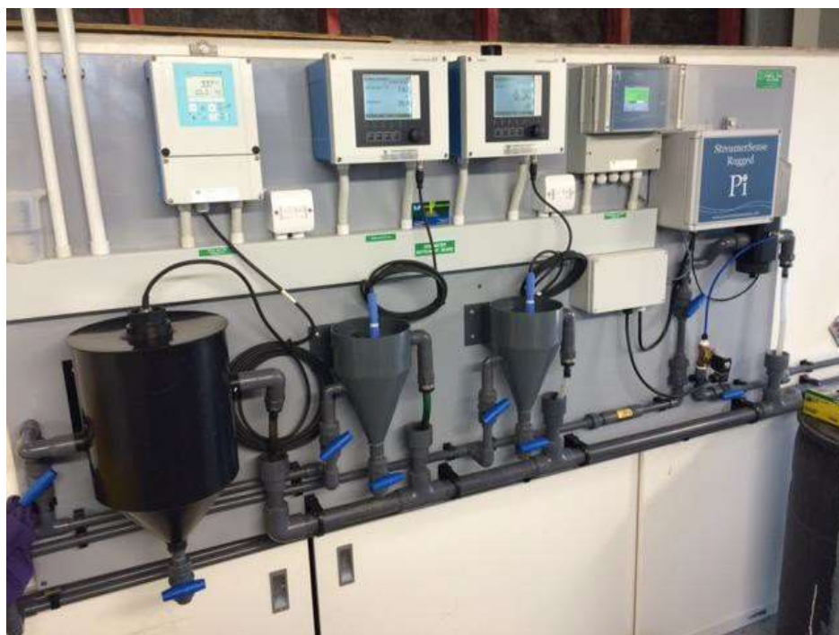
Figure 5. Coagulant Dosing Control Equipment
