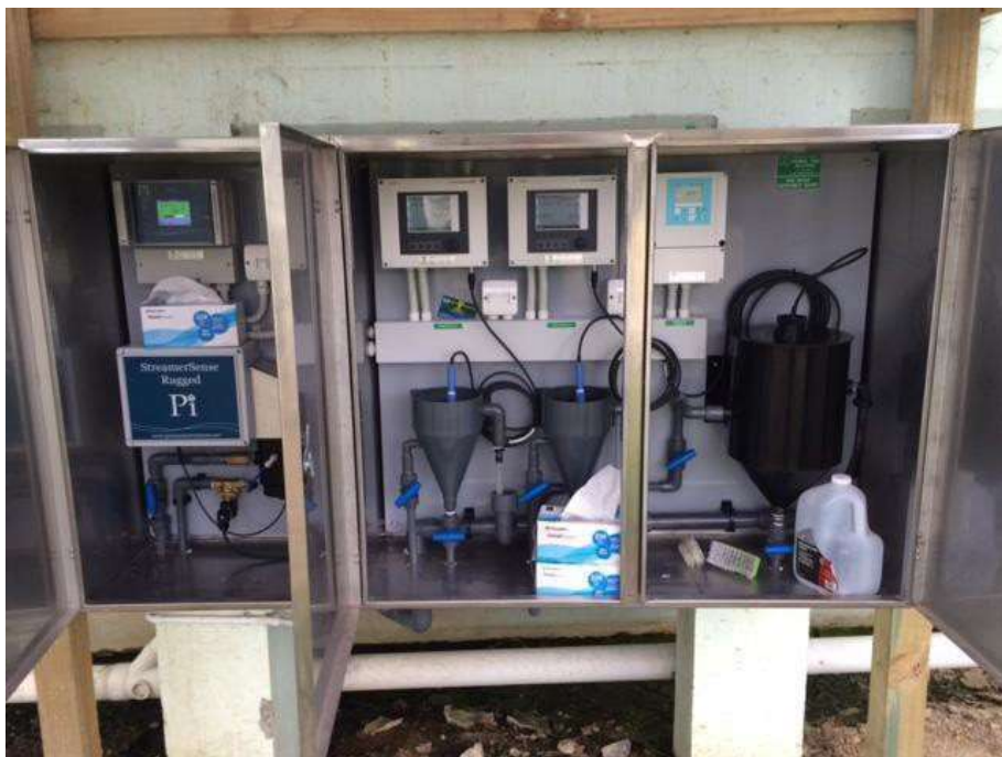
Figure 3. Coagulant Dosing Control Equipment
