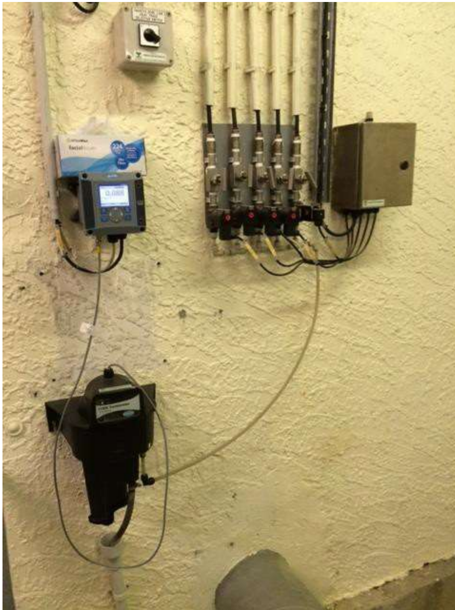
Figure 6. Clarified Water Turbidity Meter and Controls
