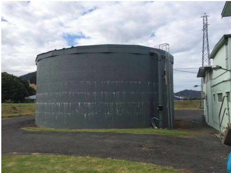
Figure 15. 900m 3 Holding Tank
