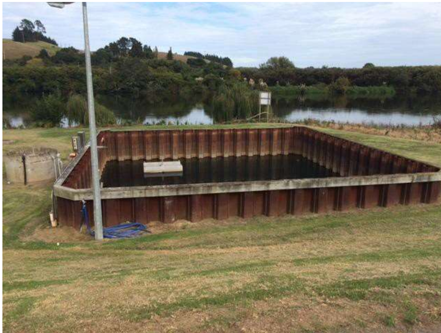
Figure 8. Clarifier and Filter Waste Settling Tank
