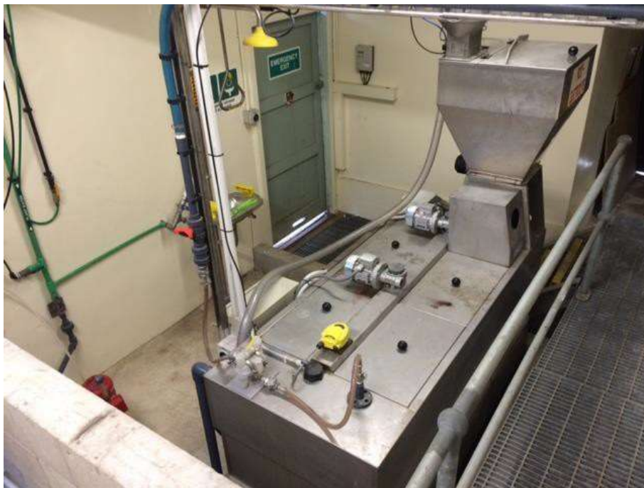
Figure 12. Poly Make-Up and Dosing Equipment
