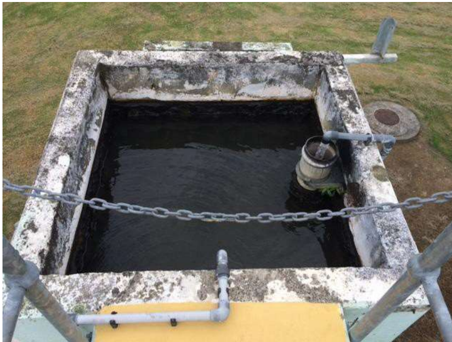
Figure 4. Flash Mixer Tank
