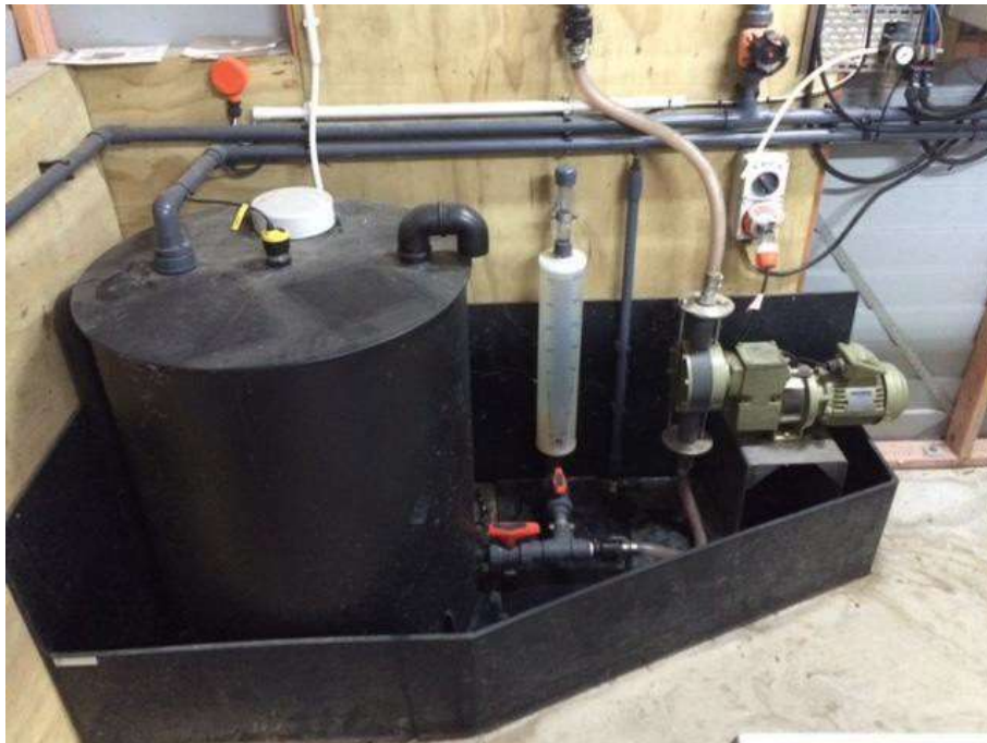
Figure 13. Fluoride Dosing Equipment
