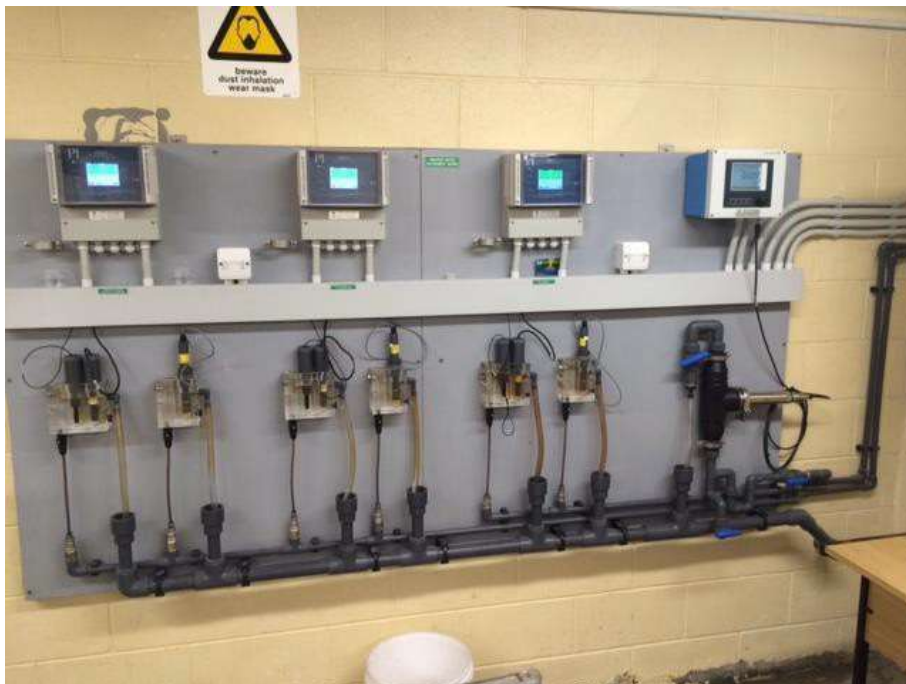
Figure 14. Final Water Quality Monitoring Instrumentation
