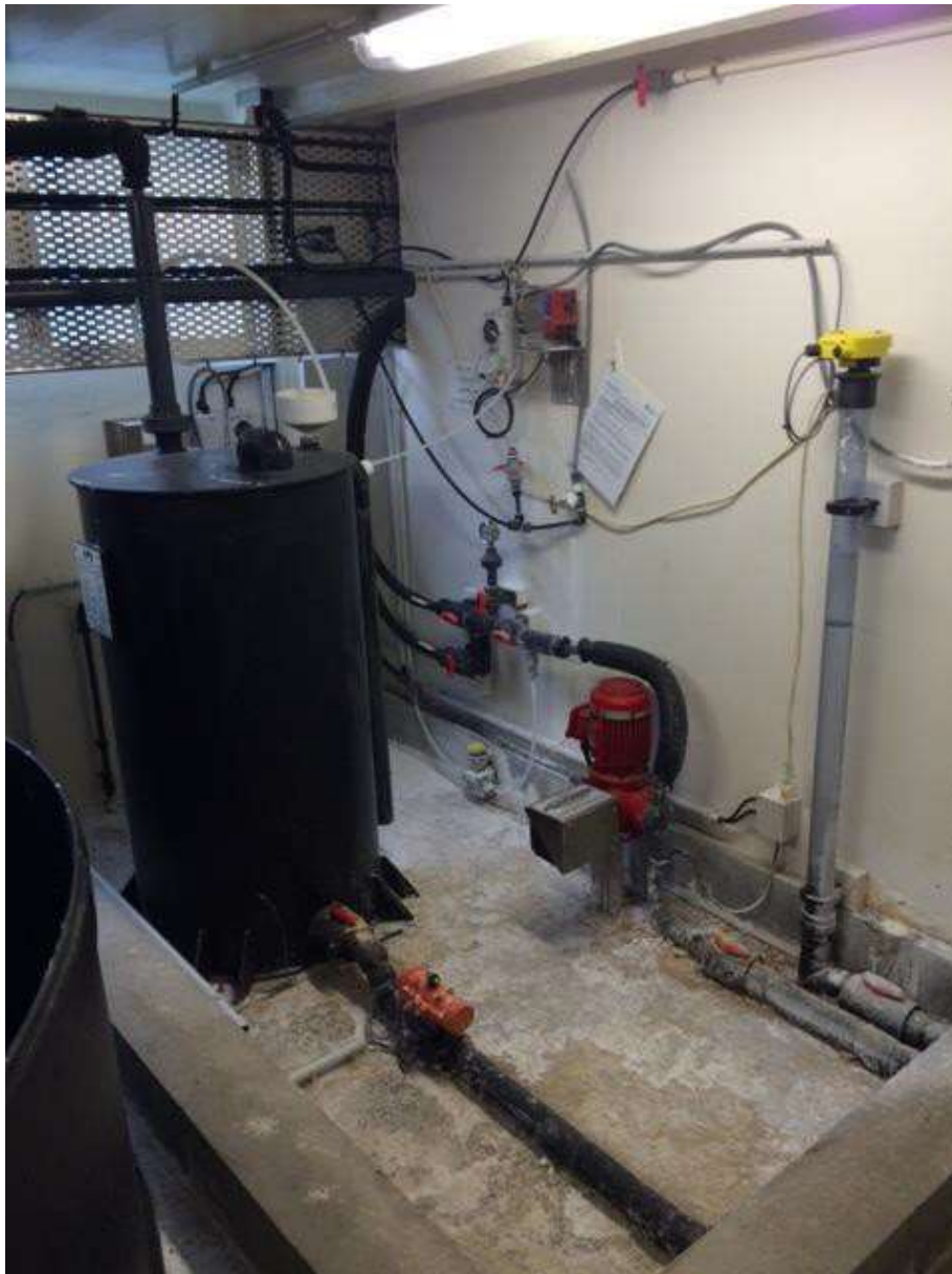
Figure 10. Caustic Dosing Equipment
