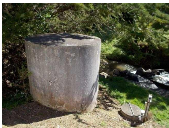
Figure 5. Raw storage and wet well
