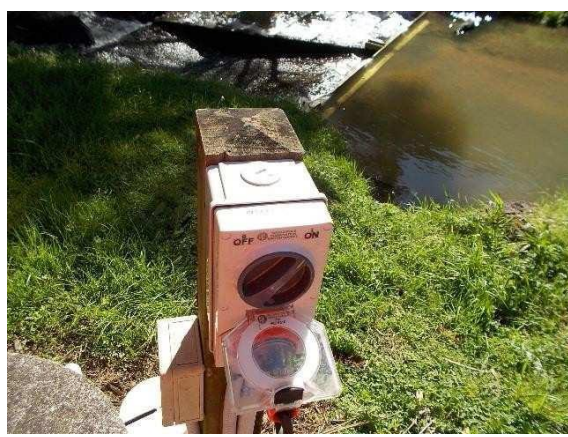
Figure 6. Abstraction pump plug and switch
