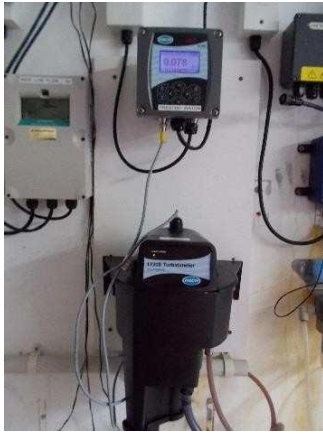
Figure 11. Post filter turbidity meter
