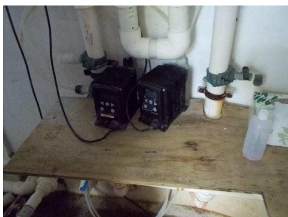
Figure 7. Soda ash and PACI dosing pumps
