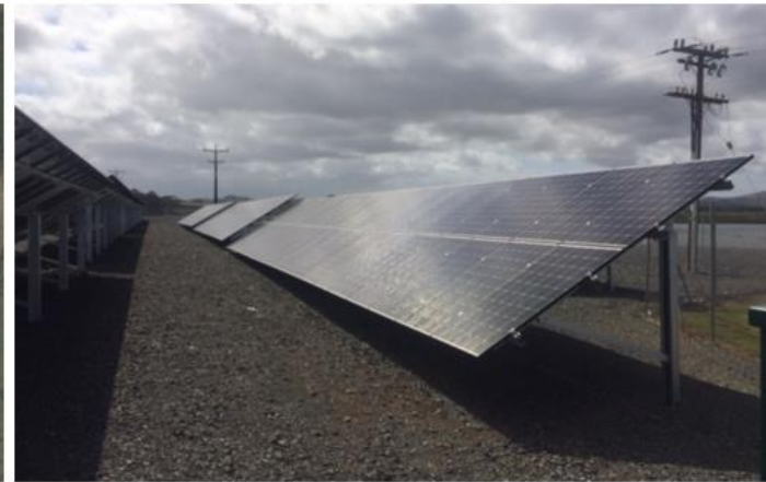
Similar ground-mounted array at Pukekohe WWTP
