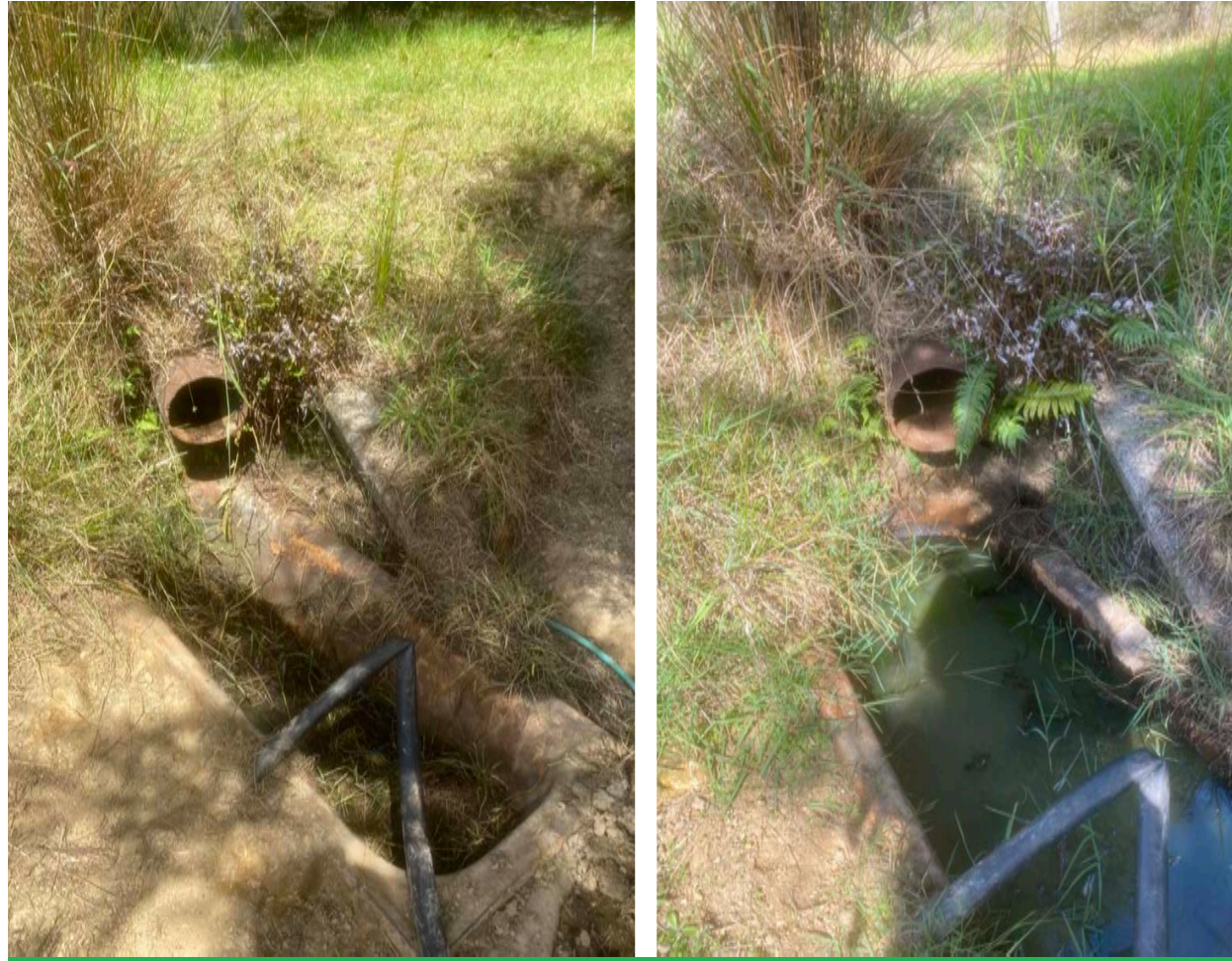
Figure 27: Perched culvert by pump shed in March 2022 (left) and May 2022 (right).
