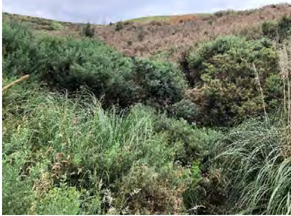
Plate 4-3: Gorse has colonised the top of the dam (looking U/S towards the pond)
