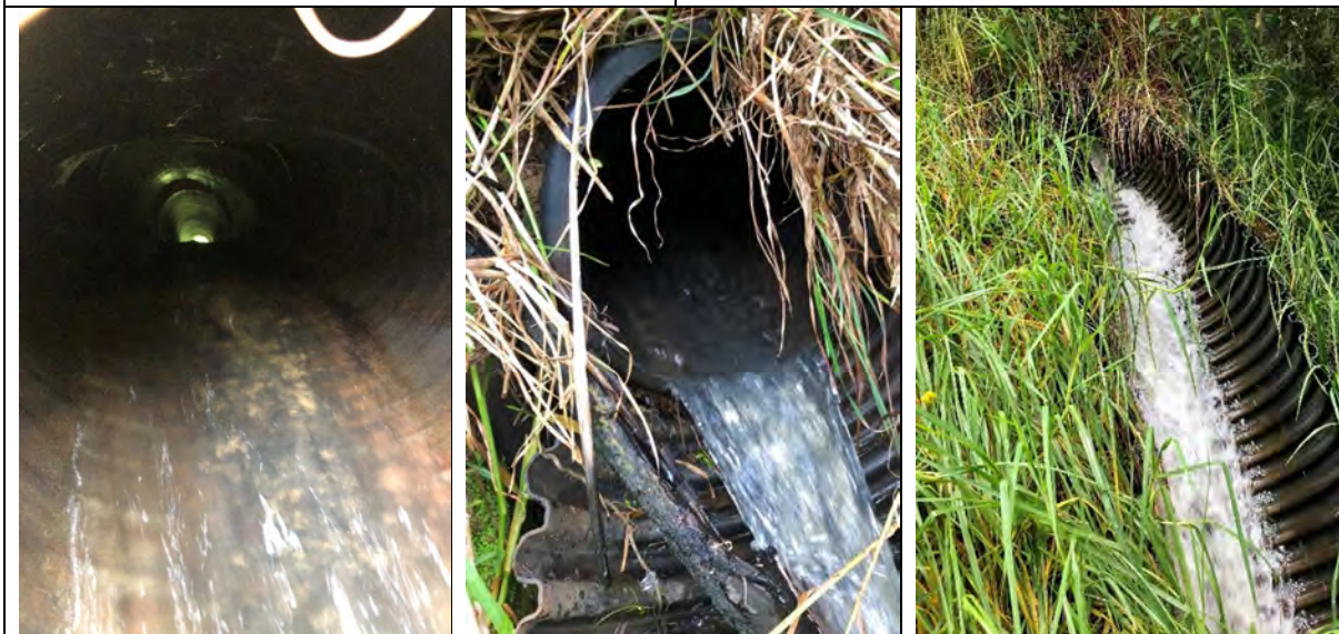
Plate 4-13a,b,c: The outlet from the pond is a culvert and half-round corrugated pipe
