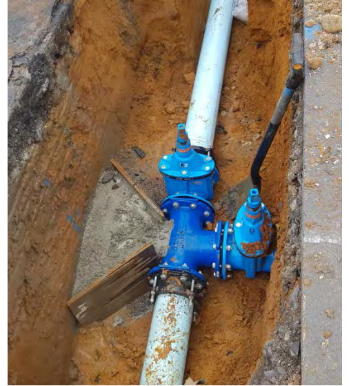
Valves and concrete thrust block
