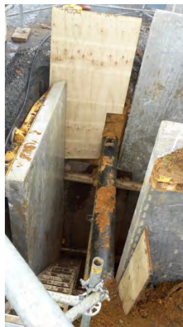
Deep excavation (4.5m) to install a gravity main and manhole around existing services
