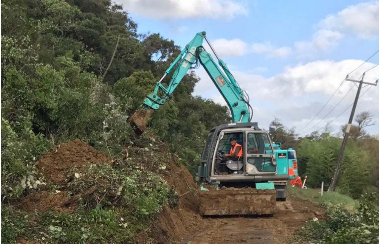
One of our HEB Supply Partner teams clearing a slip following the weather events in April.
