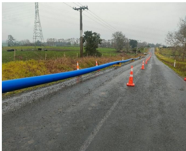
Hall Road WS Renewal – 315mm MDPE pipe drill string (200m) installed via horizontal directional drilling along with modifications to the existing network to support future connections.
