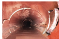
Cracked pipes like this one allow rainwater and ground water to enter the wastewater network and must be repaired.
