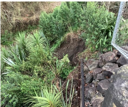
Image of the bank slippage and resultant pipe break
