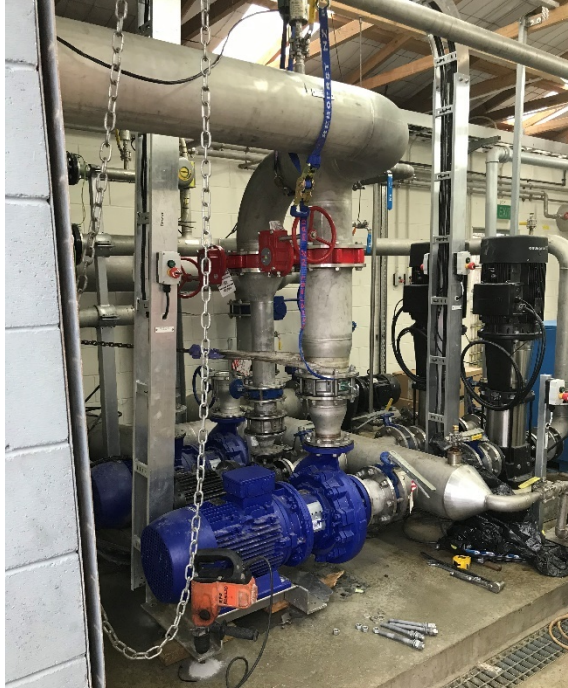
Whangamarino WTP – Upgraded Meremere and Te Kauwhata Network Supply Pumps
