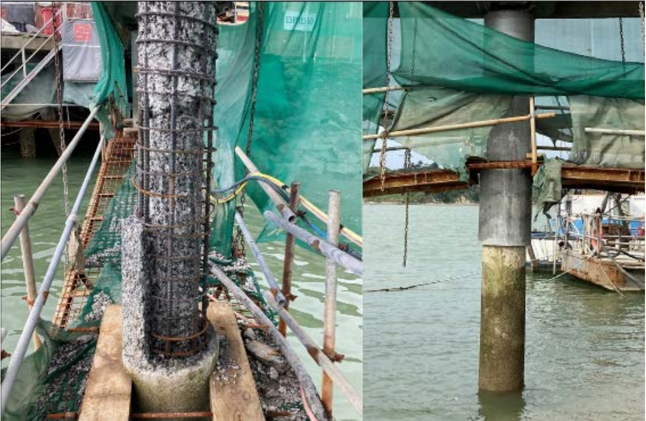
During and After of the pile repair on Dolphin Pier – note the additional cover of new concrete compared to existing.
