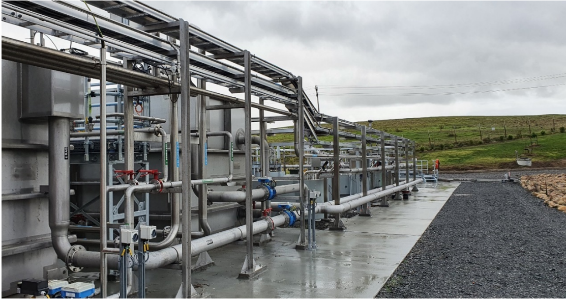
Meremere Wastewater Treatment Plant – new MBR plant
