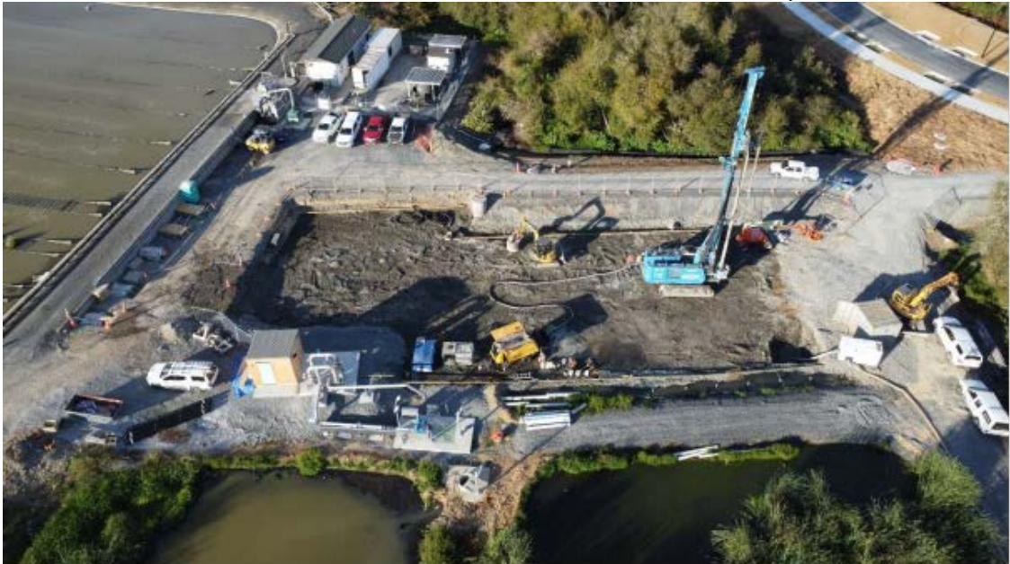
Te Kauwhata Wastewater Treatment Plant – piling works for the new MABR plant
