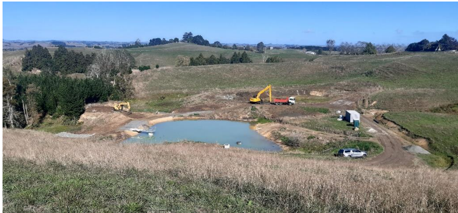
Whangamarino WTP – Pond 1 is now in service, and Desludging is underway in Pond 2
