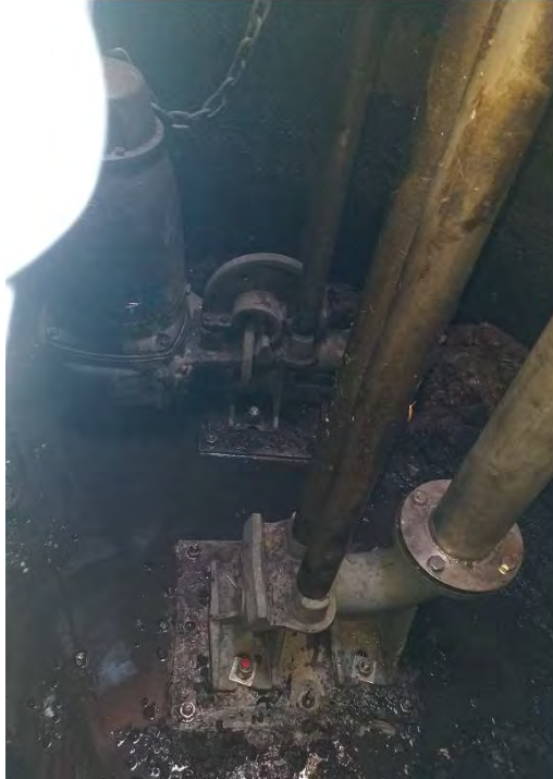
New discharge bends – Wallis St PS
