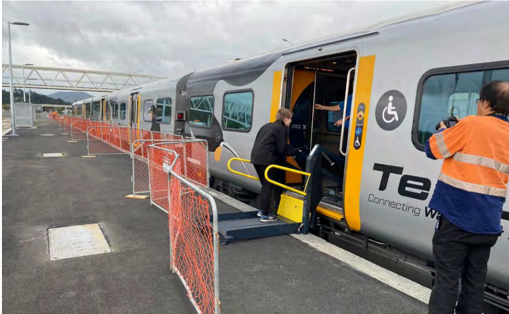
Test train at the upgraded platform checking clearances and heights – all confirmed to specification
