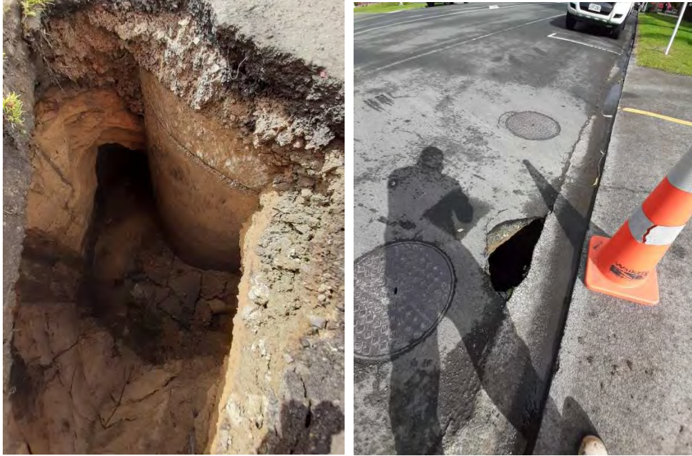
Images showing the tomo formed and collapsed roadway.
