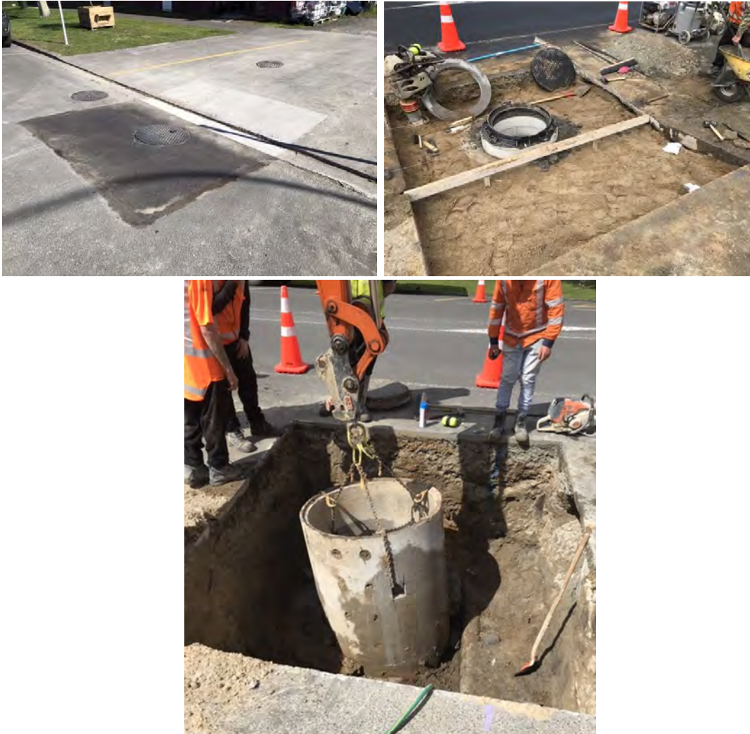
Images showing the various stages of the manhole repair at Martin St, Ngaruawahia.
