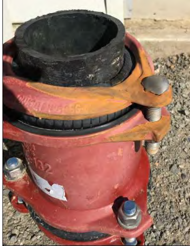
Image showing the hydraulically eroded fitting resulting in the large leak at Hampton Downs
