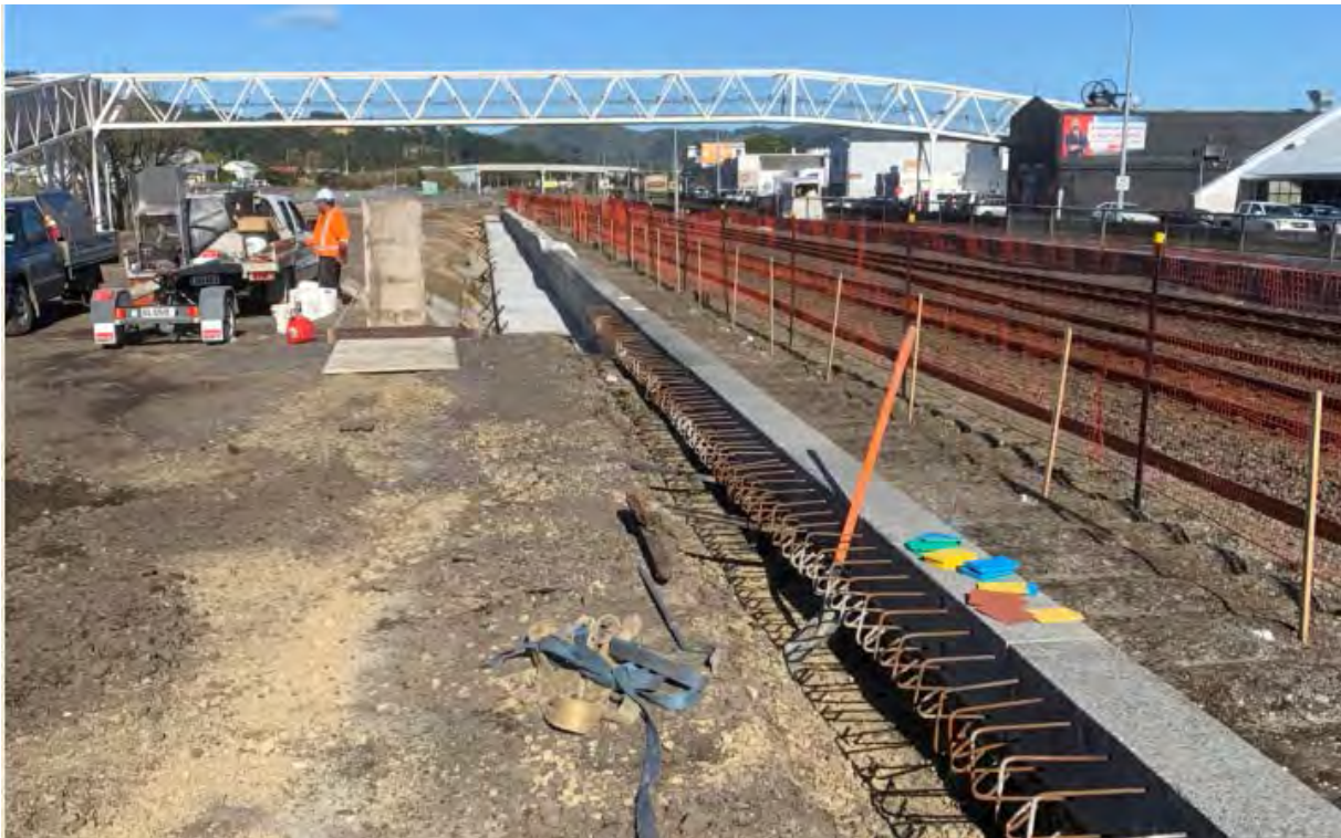
Installing new panels to raise the height of existing section of the platform to meet new standards
