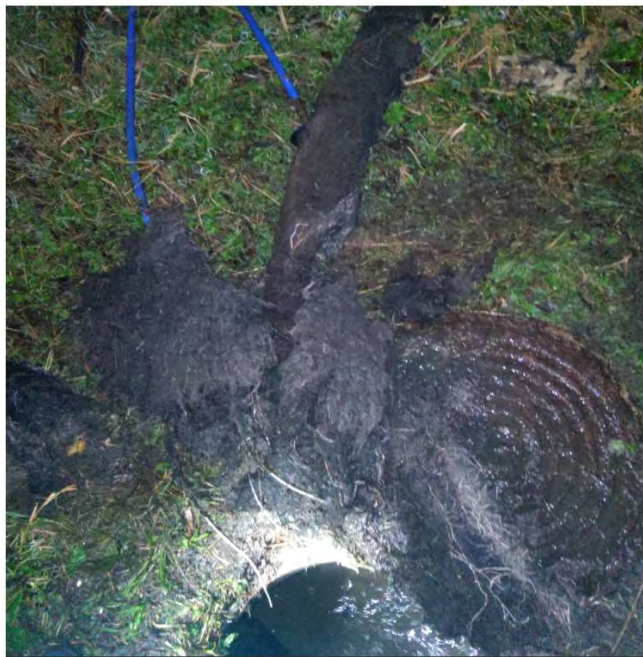
Image showing the root ball causing the blockage and resultant overflow
