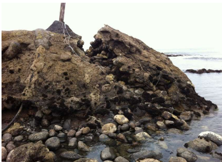
Figure 2.3. The failed tip of the old Manu Bay breakwater in late 2014.
