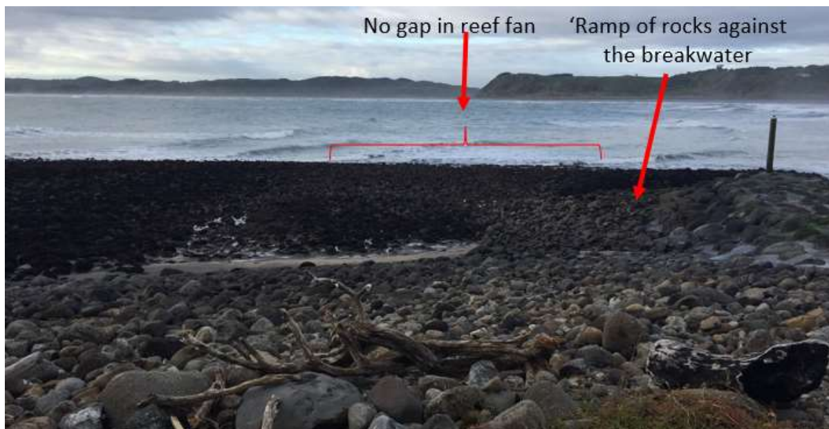
Figure 2.11. Several months after construction the scour channel that was previously present and reduced wave height at the breakwater was filled and a mound of rocks were present against the seaward side of the structure.
