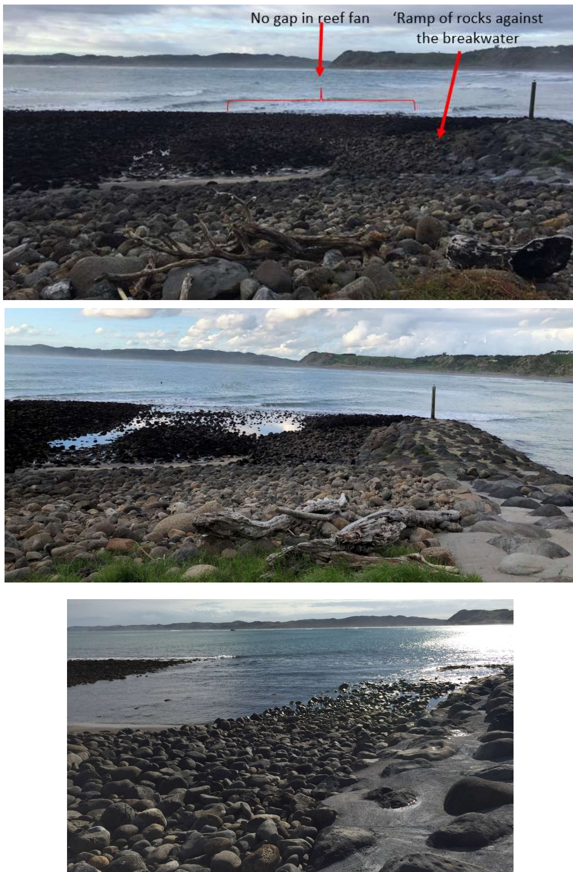
Figure 3.3. Visual evidence indicates that the scour channel on the seaward side of the breakwater is re-establishing. (Top) 3 months after construction, (Middle) late 2018 and (bottom) February 2020.
