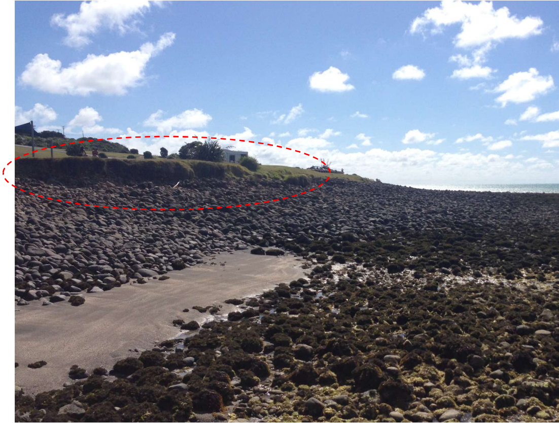
Figure 5.1. The area of chronic active erosion at the top of the foreshore on the seaward side of the breakwater.
