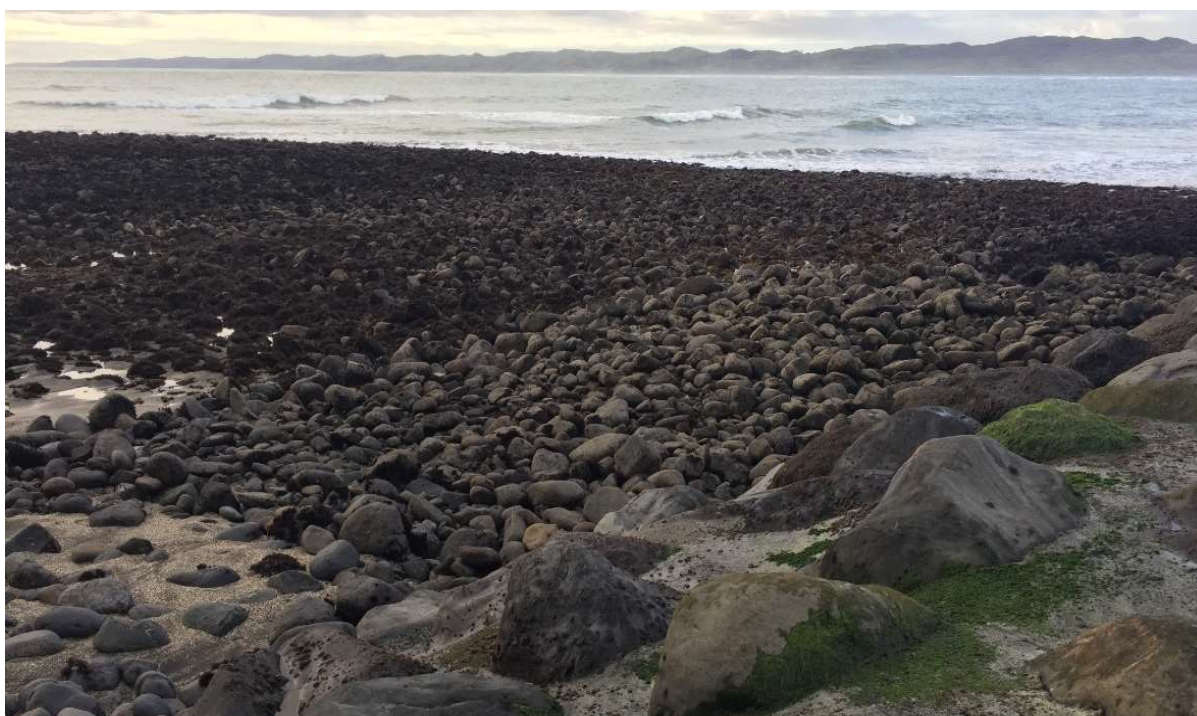
Figure 2.12. The mound of rocks post-construction where there was formally a scour channel allow waves to shoal all the way to the breakwater with more potential for over-topping.
