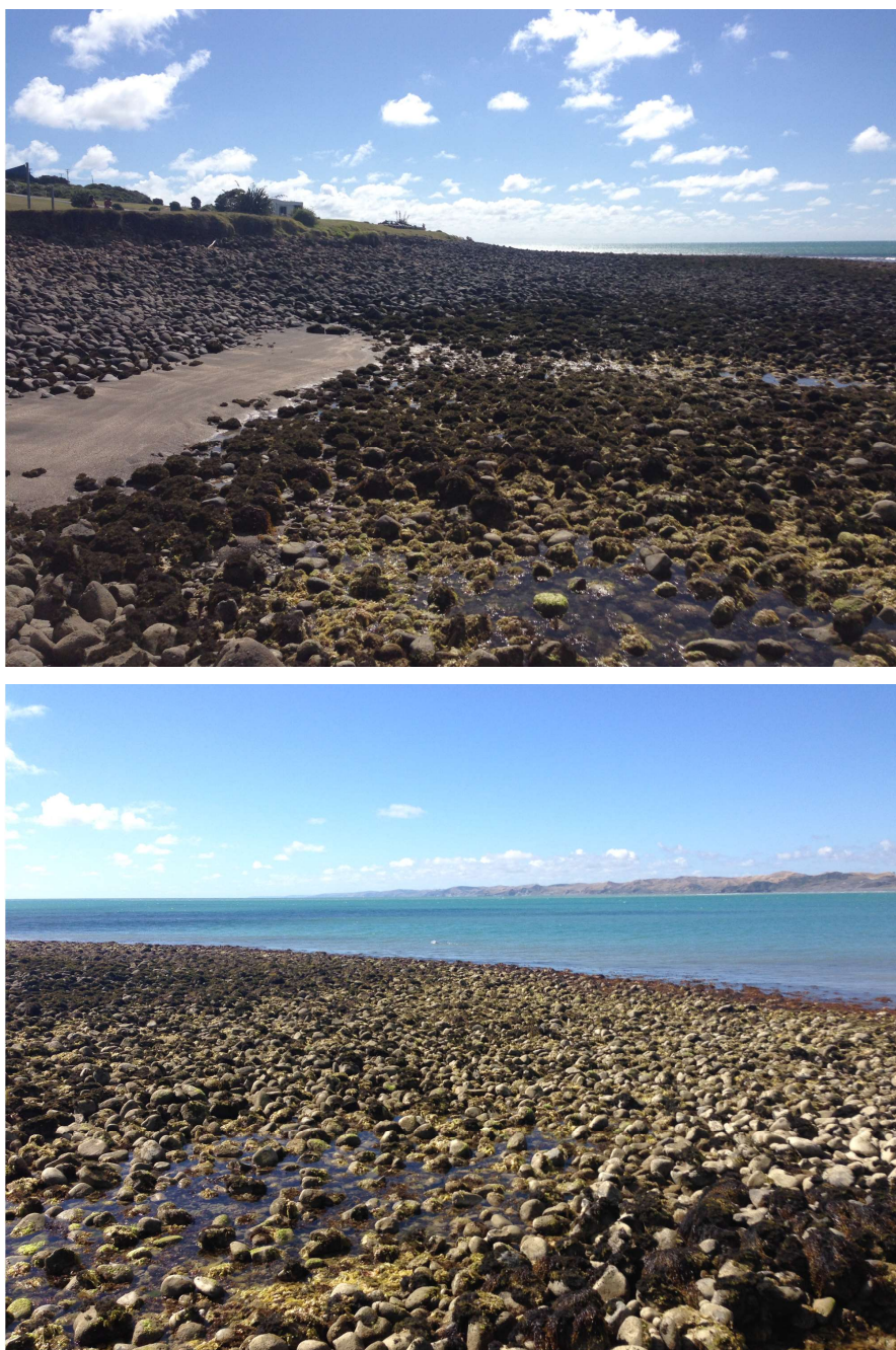
Figure 2.9. Before the construction of the new breakwater, a significant scour channel was present on the northern side of the breakwater, which can be seen here with lighter coloured seaweeds and a strip of sand at the landward end – also see Figure 2.1, Figure 2.2 and Figure 2.10.
