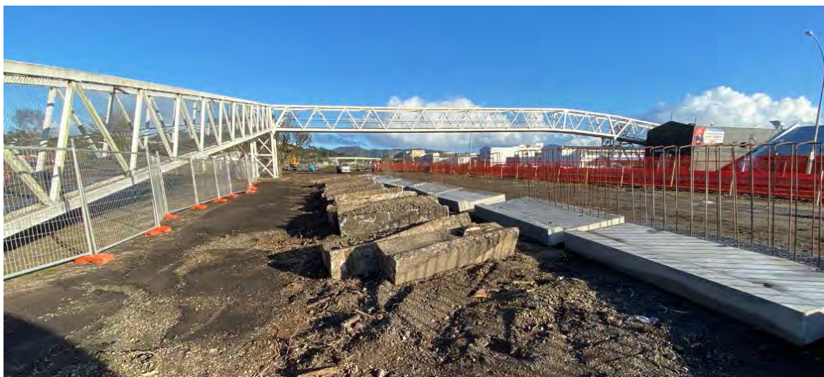
Old demolished platform wall units and the new precast units ready to be placed.
