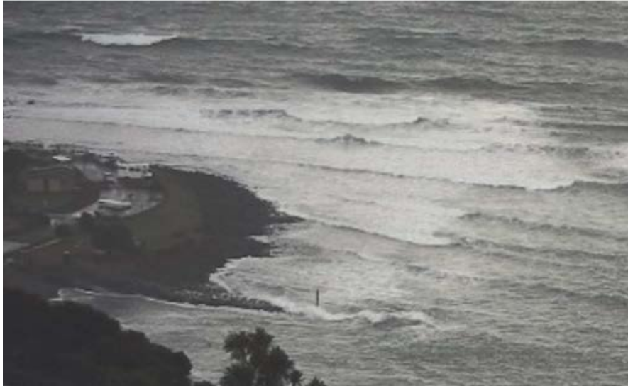
Overtopping of Manu Bay breakwater in mid-2019
