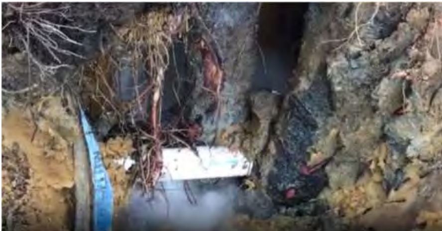
Location of break @ Springhill Rd – note the root damage
