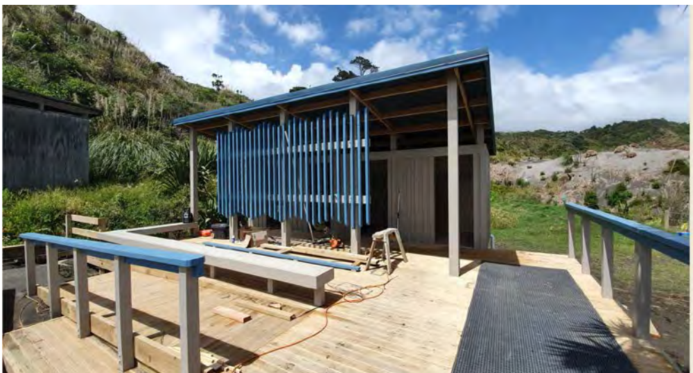
Progress Photo – 15 Nov. Work remaining is 2nd fix plumbing, shower install, asphalt access works
