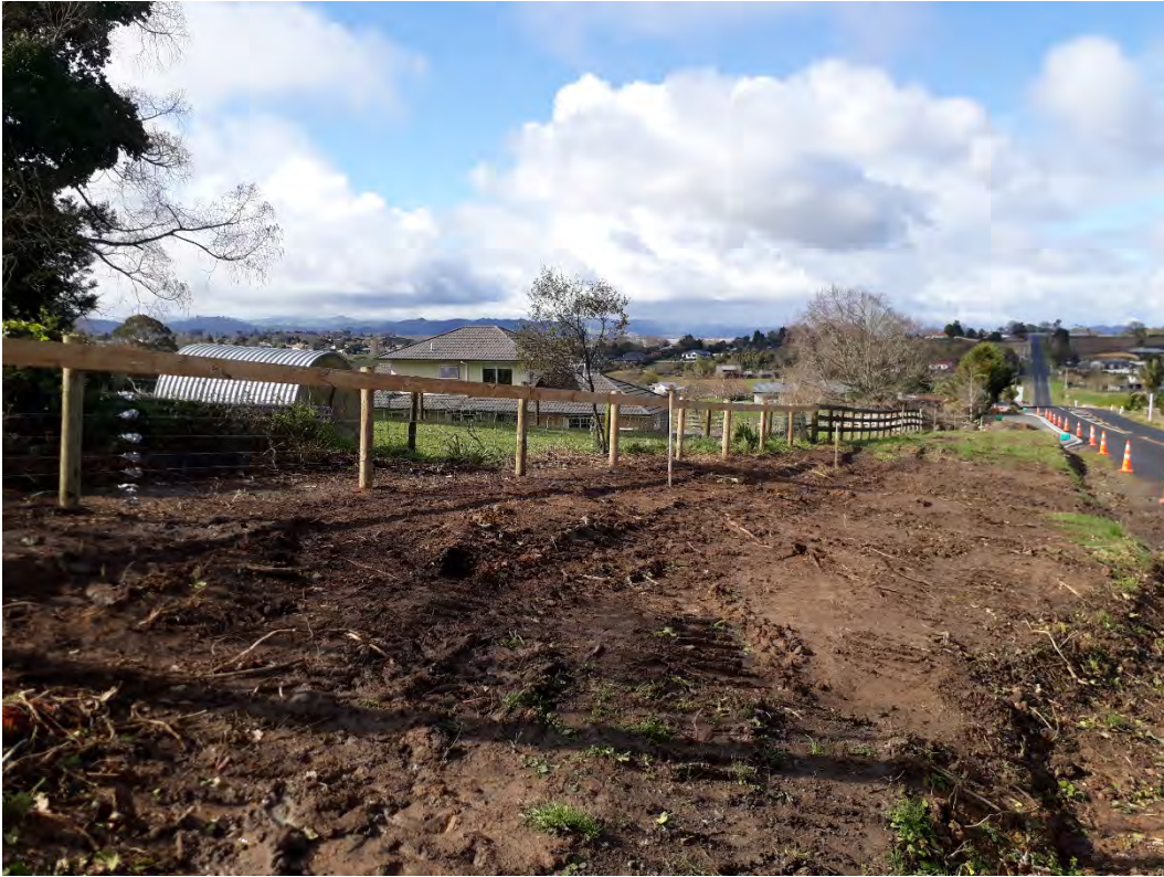
Progress Photo of fencing and formation works required immediate near Moorfield Rd – 23 August 2019
