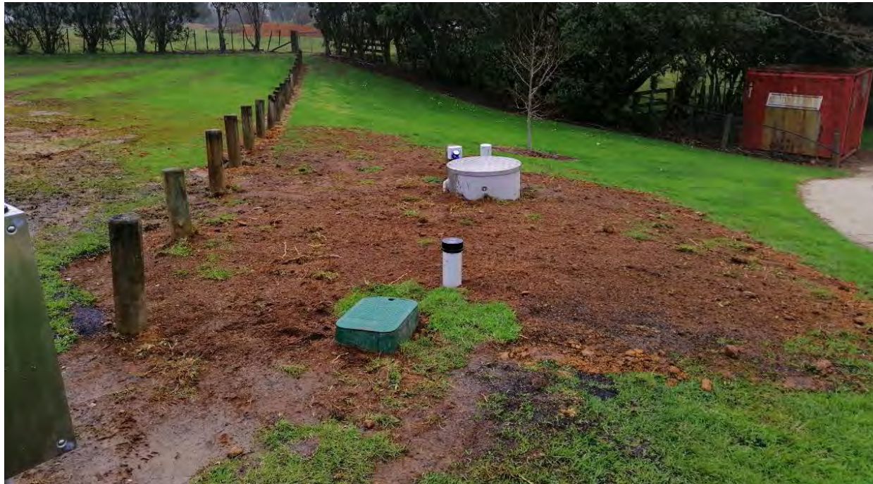
Buffer tank installed
