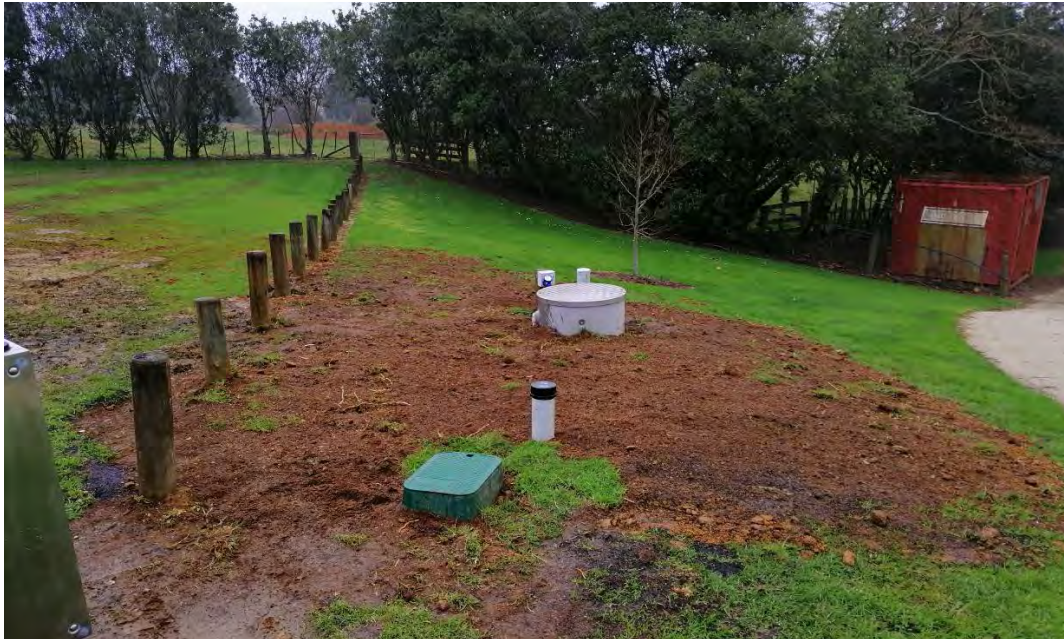
New 25,000 litre buffer tanks and monitoring system
