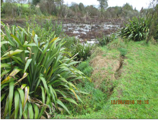
Slumping of existing track outside of Lot 20
