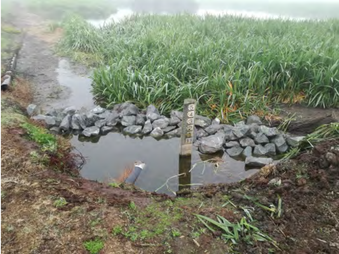
Huntly Wastewater Wetland
