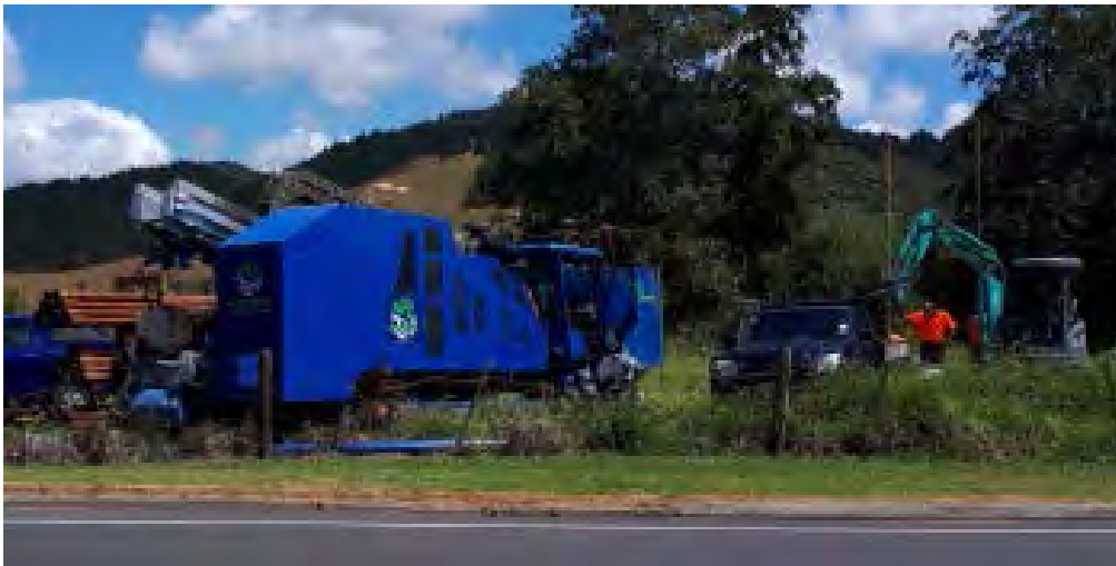
Drill rig on site for installing pipe under the Waikato River at Taupiri. Will move to Tuakau when complete
