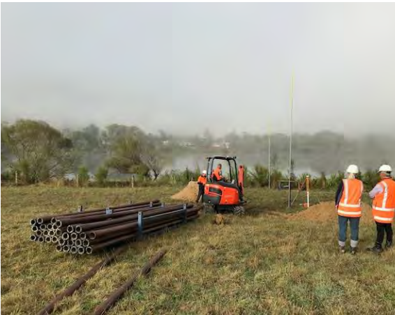
Northern River Crossing preparing for pilot drill shot to break through (Observed by Archaeologist, Alexy Simmons, and WDC Iwi & Community Partnership Manager, Sam Toka.
