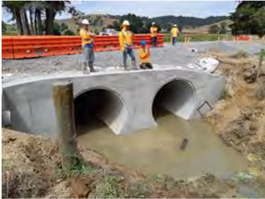
Dimmock Road Culvert Installation (Prior to dirty water being pumped from closed off area)
