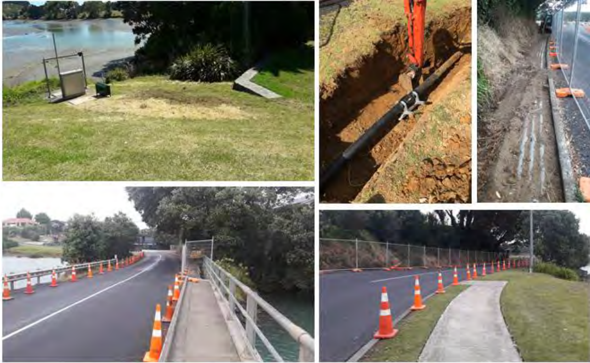
Completed rising main replacement at Nihinihi Avenue Pumpstation, along with construction progress photos with completion of the second section at Marine Parade
