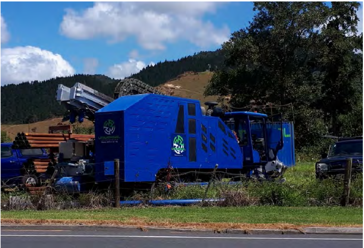
200 ton pull capacity drill rig (one of only four this powerful in the country) - currently in Taupiri – will then head to Tuakau
