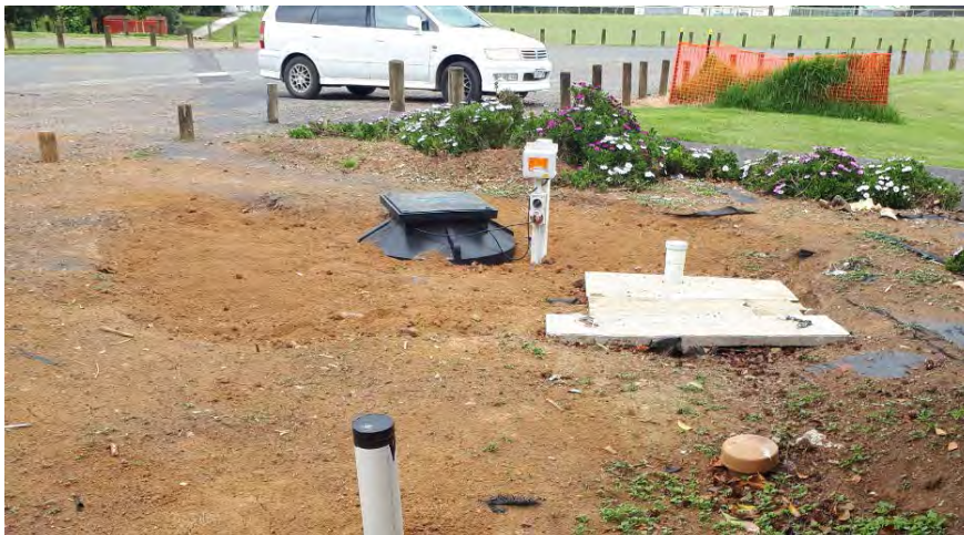
Existing septic tank with new pump and filter
