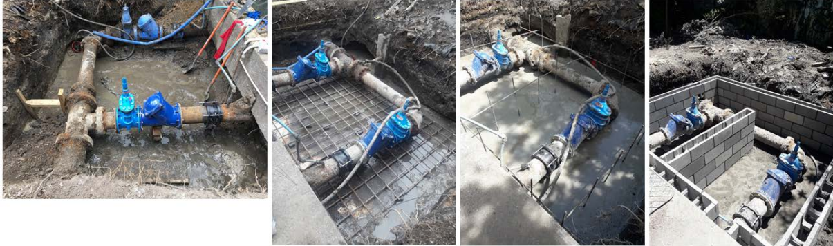
WDC wastewater pumpstation located within the grounds of Huntly Primary School – non-return valve and isolation valve replacement with a full valve chamber construction in progress
