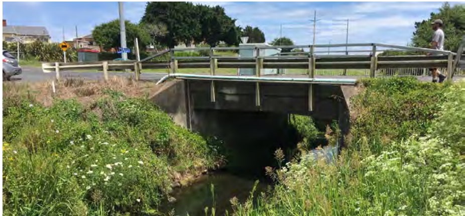
View of potential footpath stream crossing from upstream on right stream bank (note pedestrian crossing the bridge in the live traffic lane).
