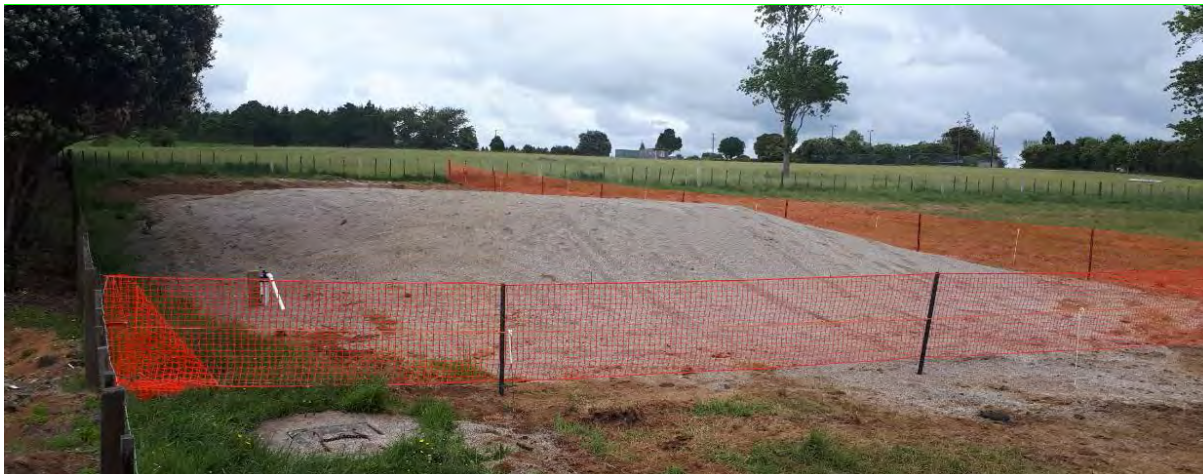
Wisconsin Mound for effluent soakage and evaporation
