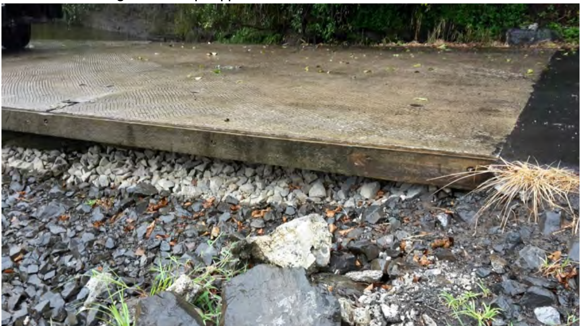
Undermining of Narrows Boat Ramp
