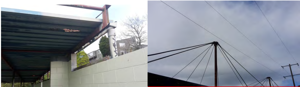
Grandstand Roof – overhead electrical wires an added safety component
