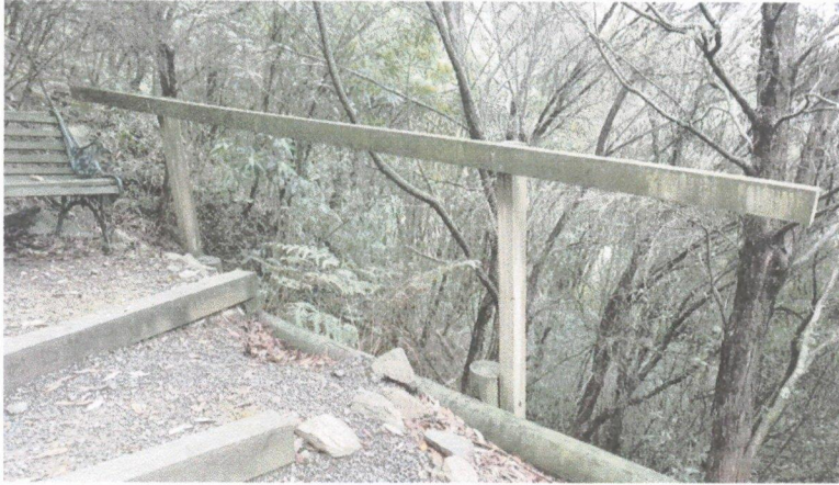
Photo 6: unsafe rail (G21 on map)
