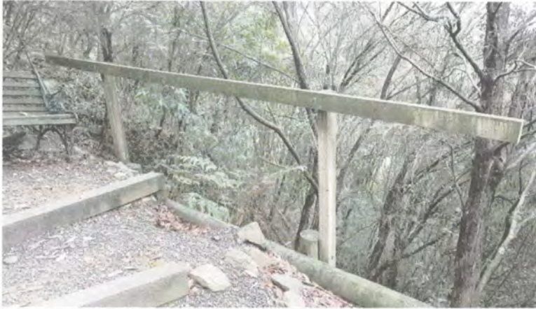
Photo 6: unsafe rail (G21 on map)
