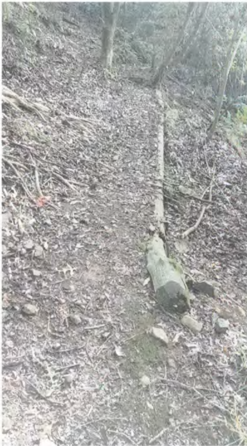
Photo 4: rotten retaining timber, sloping track and bank down to pond
