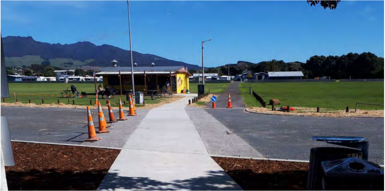
Papahua – Car Park Upgrade Works feature a new extended path and raised crossing
