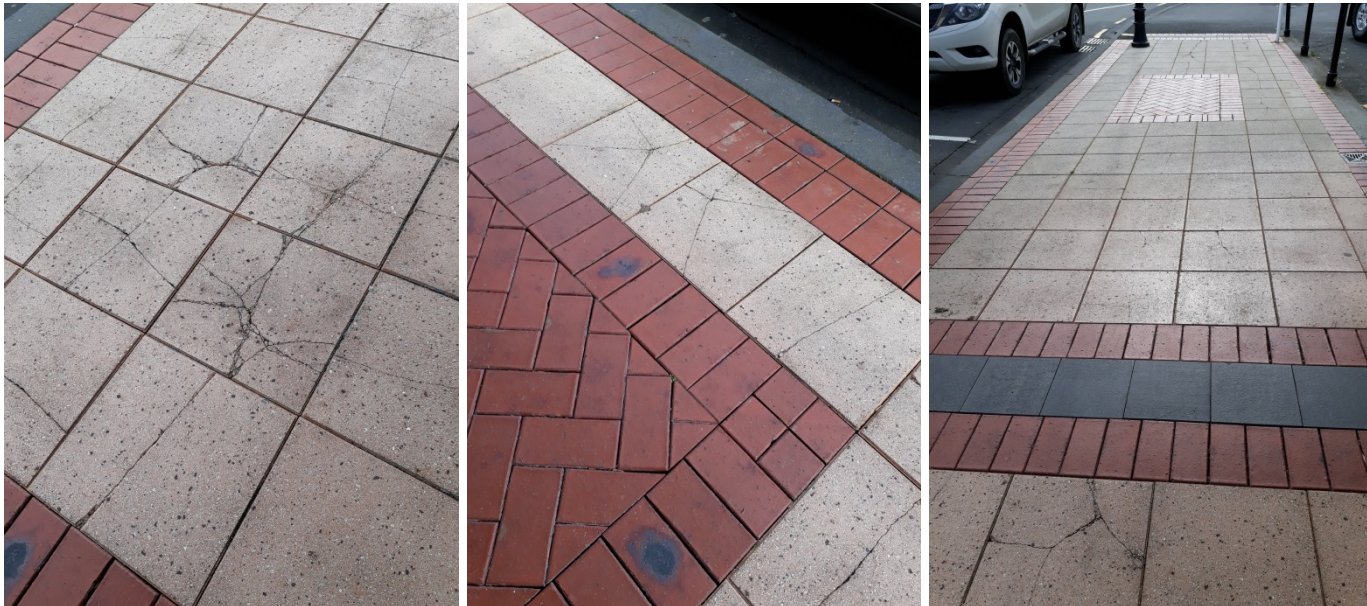
EXAMPLES of broken pavers outside of Fruit King (55 Main Street)
