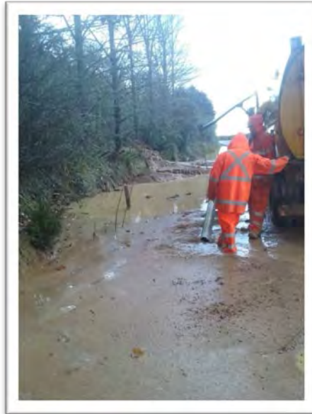
Falls Road Slip Material
