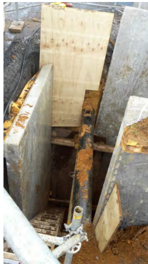
Deep excavation (4.5m) to install a gravity main and manhole around existing services
