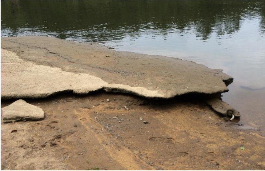
Figure 5: Undermining at the end of the Les Batkin Reserve Secondary Boat Ramp, Waikato River.
