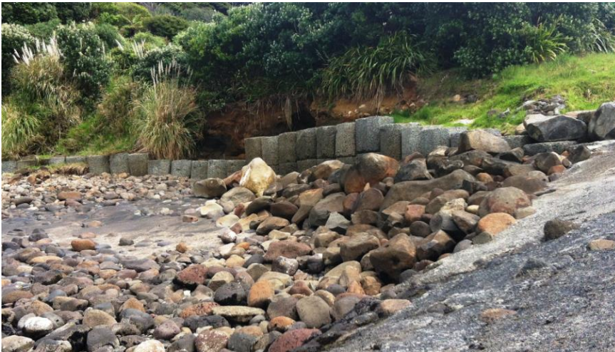
Figure 15: Area of erosion and subsequent erosion protection wall installation adjacent to Manu Bay Boat Ramp.
