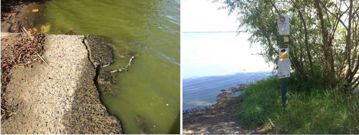
Figures 26 & 27: Existing concrete ramp with end breakage effects and signage at the additional ramp within the Waikare Reserve.
