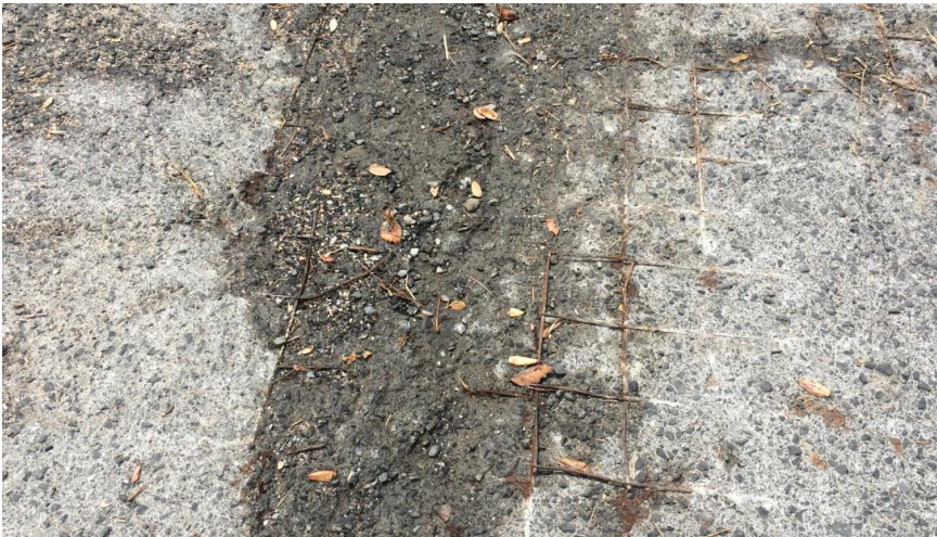
Figure 10: Surface wear on the Wallace St Boat Ramp, Whaingaroa Harbour resulting in uneven surfaces and exposure of steel meshing.
