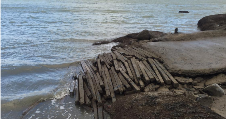
Figure 20: Poor boat ramp design and end break age effects resulting in ad hoc public works to extend the Te Akau boat ramp.
