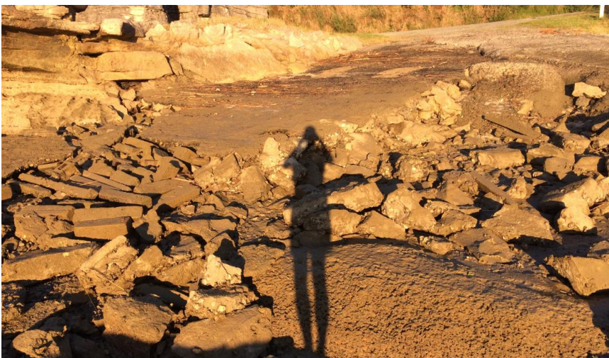
Figure 18: Deposition of concrete rubble from the degraded former Te Akau Boat Ramp, Whaingaroa Harbour.
