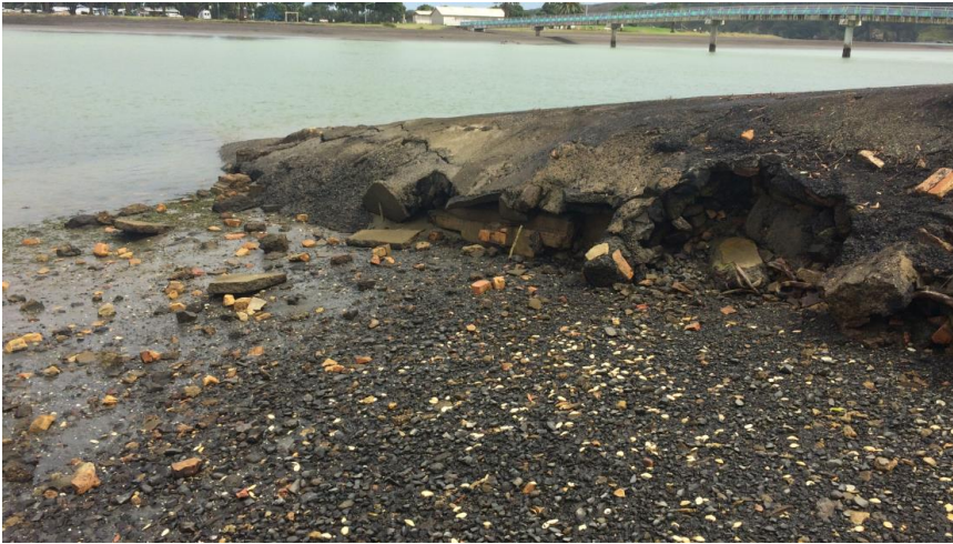
Figure 16: Deposition of boat ramp construction rubble (gravel/bricks/concrete) upon the adjacent mud/sand flats following undermining of the Raglan Coastguard Boat ramp, Whaingaroa Harbour.
