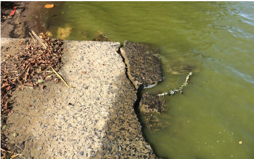
Figure 8: End breakage at the Lake Waikare Boat Ramp, Lake Waikare.
