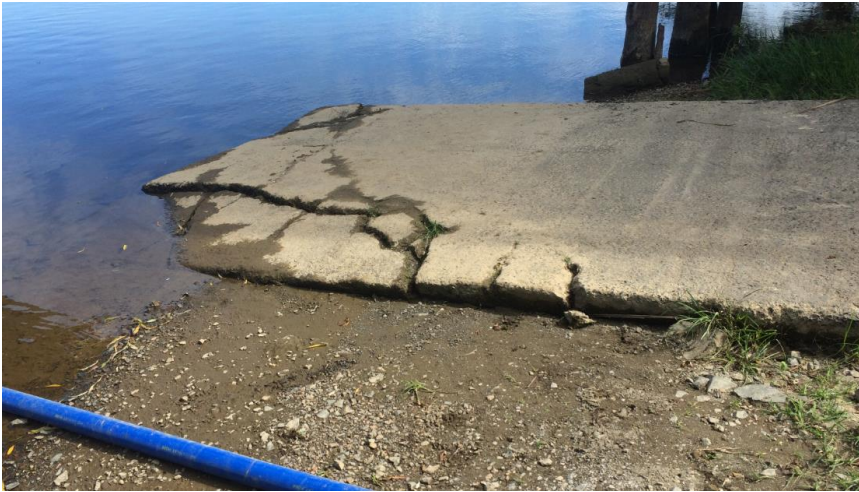
Figure 7: End breakage at the Rangiriri Boat Ramp, Waikato River. Possibly due to this ramp being used by heavy vehicles as a construction water take site during the construction of the Rangiriri Section of the Waikato Expressway.
