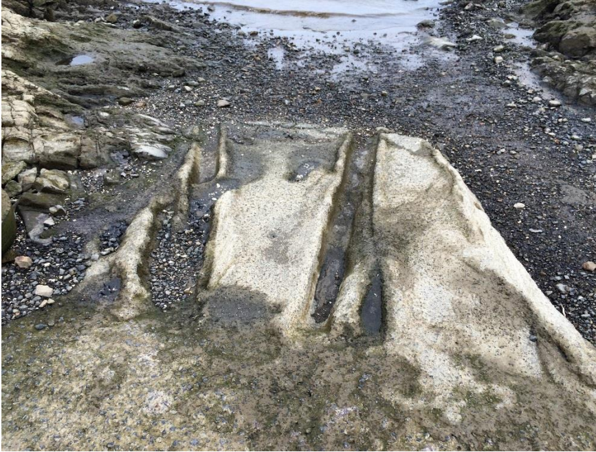
Figure 22: Uncontrolled concrete pour to extend the end of the Port Waikato Esplanade North ramp.
