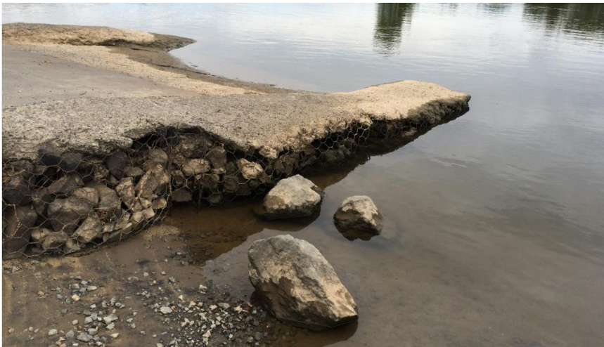
Figure 17: Deposition of quarried boulders and gravels onto the river bed following undermining of the Mercer Boat Ramp, Waikato River.
