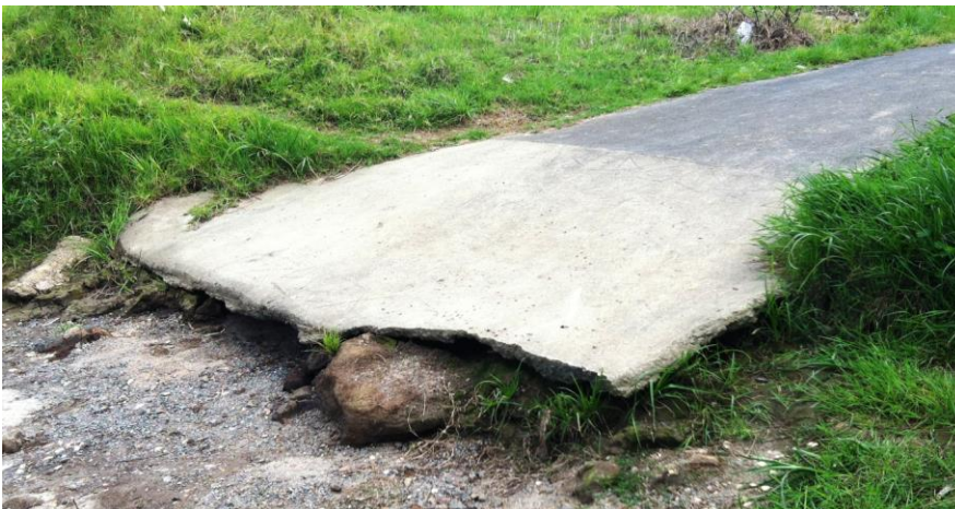
Figure 6: Undermining at the end of the Taupiri Boat Ramp, Waikato River – prior to recent repair.
