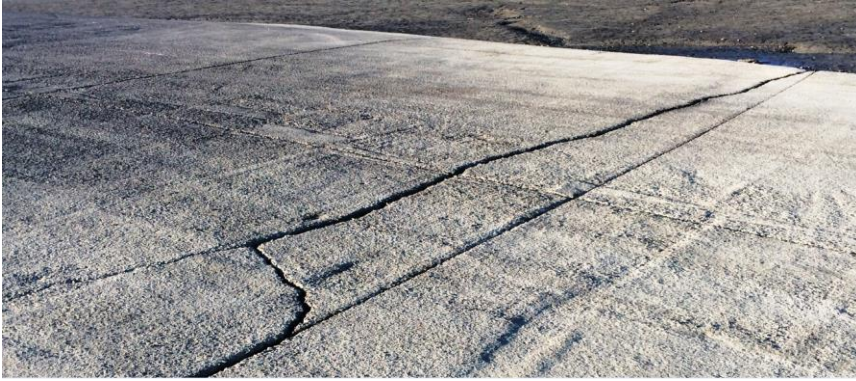
Figure 9: A large crack forming in the Kopua Domain Boat Ramp, Whaingaroa Harbour, due to undermining effects.
